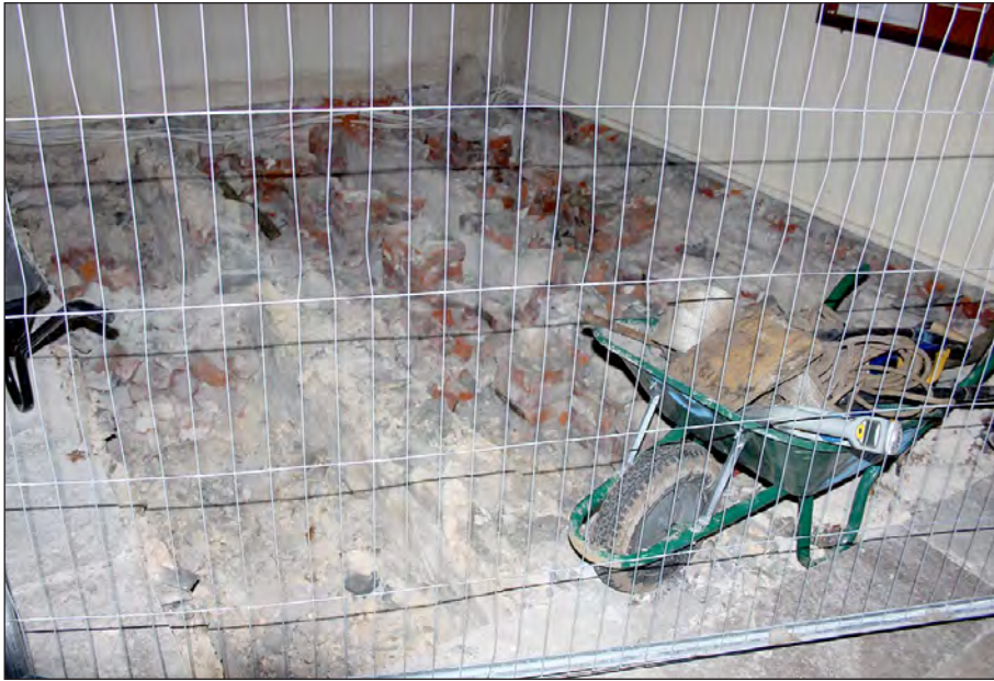
Plate 15: View of working area following the lifting of flooring slabs within the church
