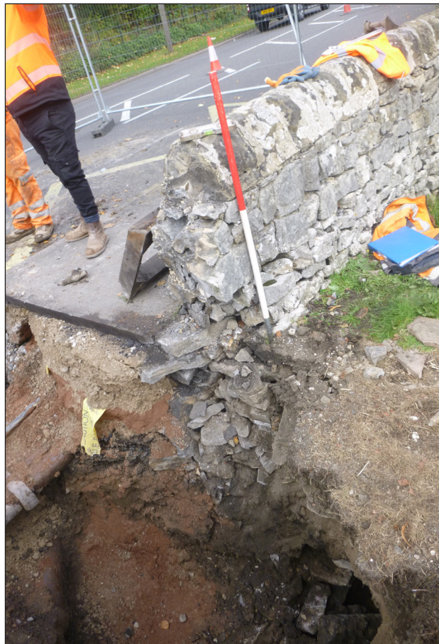
Figure 6: View from the south-east of culvert 1006 (bottom of the photo), associated with canalised stream and upstanding wall 1005 (1 m scale)
