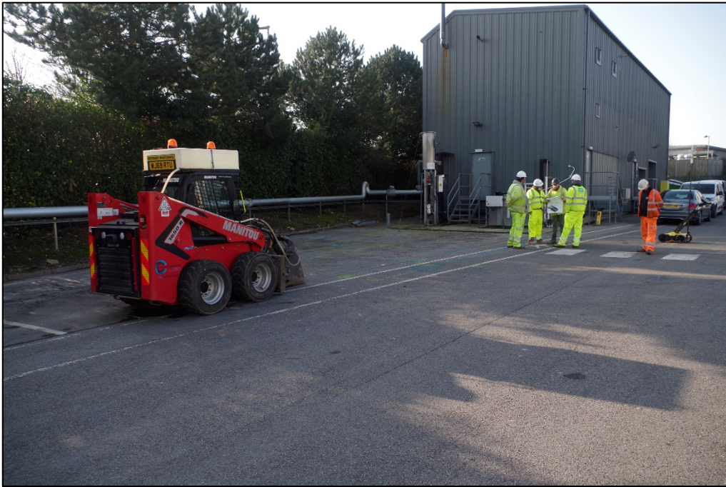
Plate 1: General view of the Site location, pre work commencement. View from the south.
