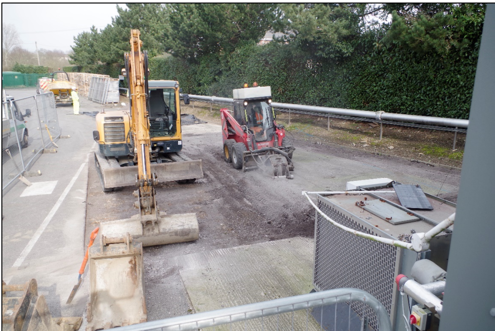
Plate 2: General view of the removal of tarmac and start of the works. View from the Northeast.
