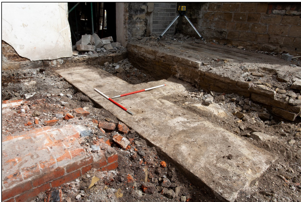
Plate 14: Exposed machine bases / engine bed (2007) within the southeast of Building 11, facing east
