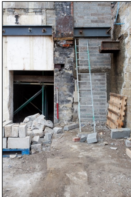
Plate 18: The former void area to the south-eastern end of Building 11, facing northeast. Note the remnant ironwork in the location of the removed dividing wall and to the top right
