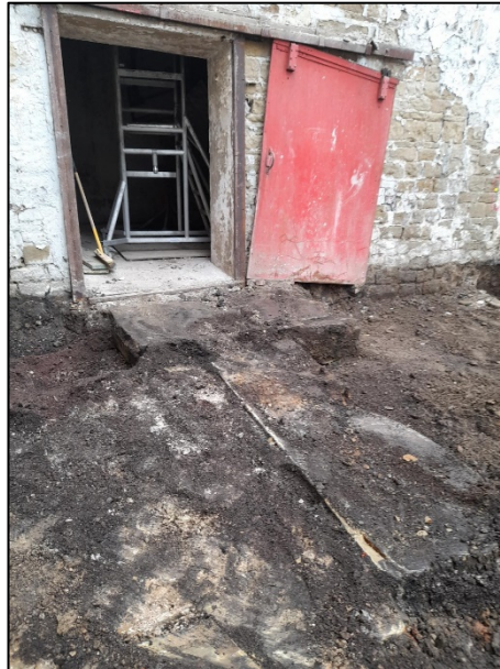
Plate 7: Client photograph 7, showing excavations within the southwest end of Building 10, revealing large stone machine beds adjacent to the doorway to Building 11, facing southwest
