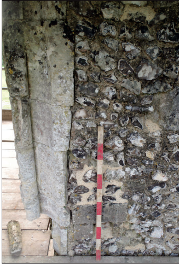
Plate 43: New crack in Great Hall, West Tower end from the west (1m scale)
