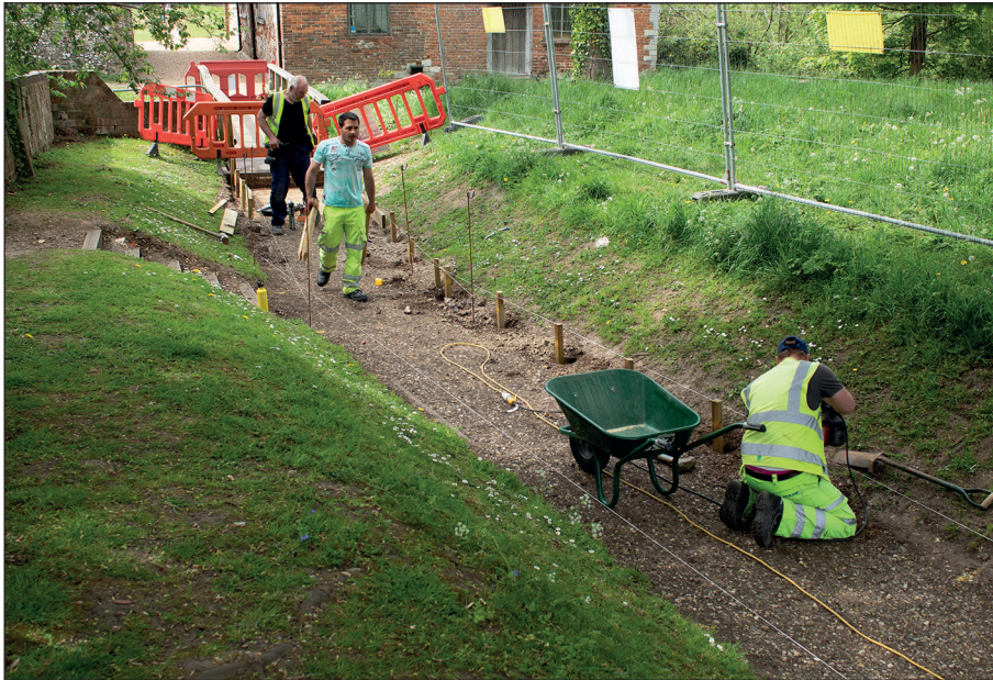
Plate 9: Removal of path surface and installation of wooden edging, view from the north-west
