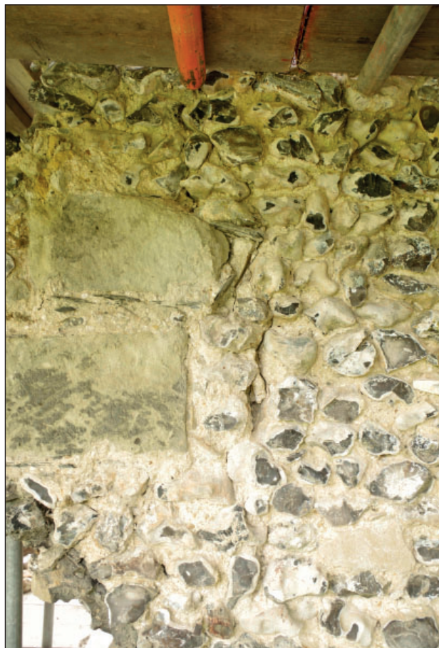
Plate 36: Crack in north wall of Kitchen from the north
