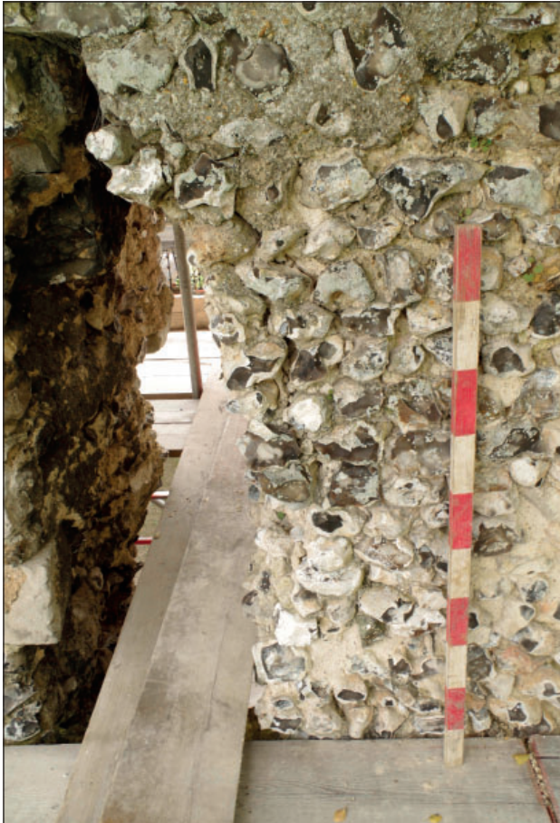
Plate 37: Significant fracture in north wall of Kitchen from the north (1 m scale)
