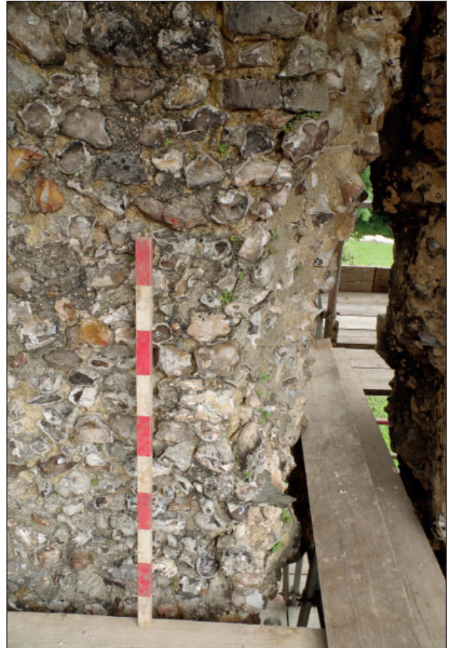
Plate 38: Significant fracture in north wall of Kitchen from the south (1 m scale)
