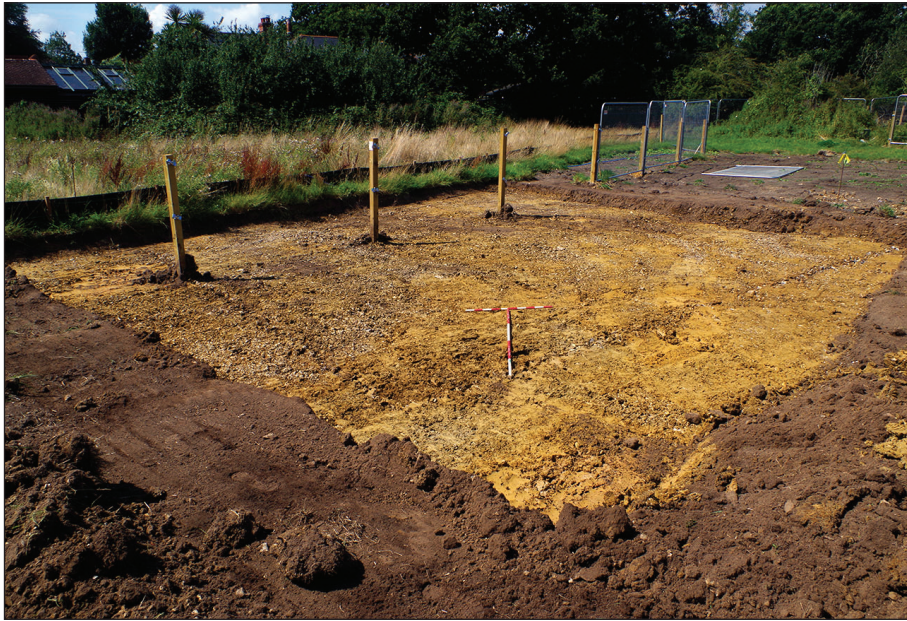
Plate 3: Example of blank area, South-East facing Area 3, with French drain, 1 x 1 m and 1 x 2 m scale
