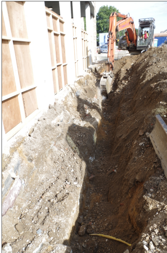
Plate 12: Service trench showing natural gravels directly beneath previous development, viewed from the southeast
