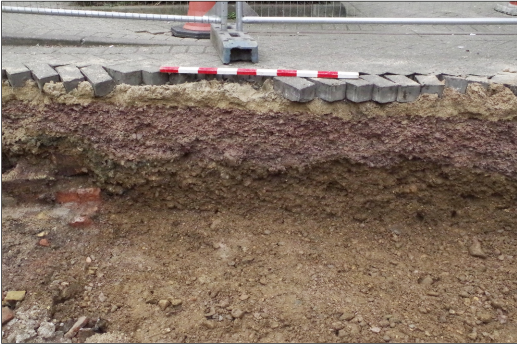
Plate 5: Representative section of Trench 2 viewed from the west showing surviving natural gravels
