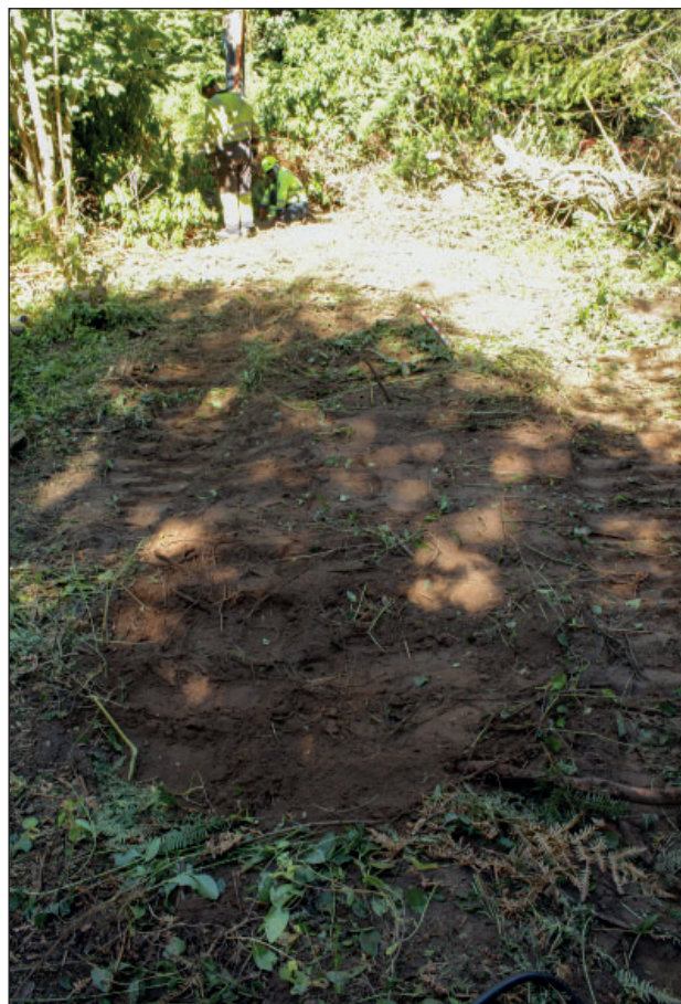
Figure 20: Backfilled area at Location 3, view from the south-east
