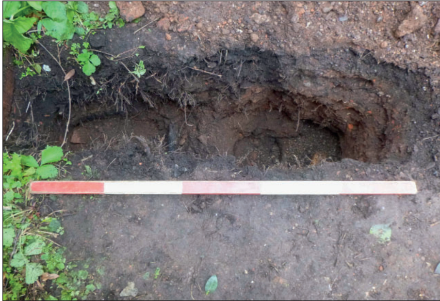
Figure 6: TP7, modern services, 1 x 1 m scale
