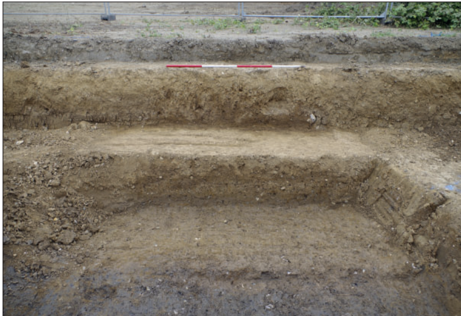
Figure 4: West facing stepped section for southern cofferdam, 2 m scale. (Photograph taken by Lisa McCaig)
