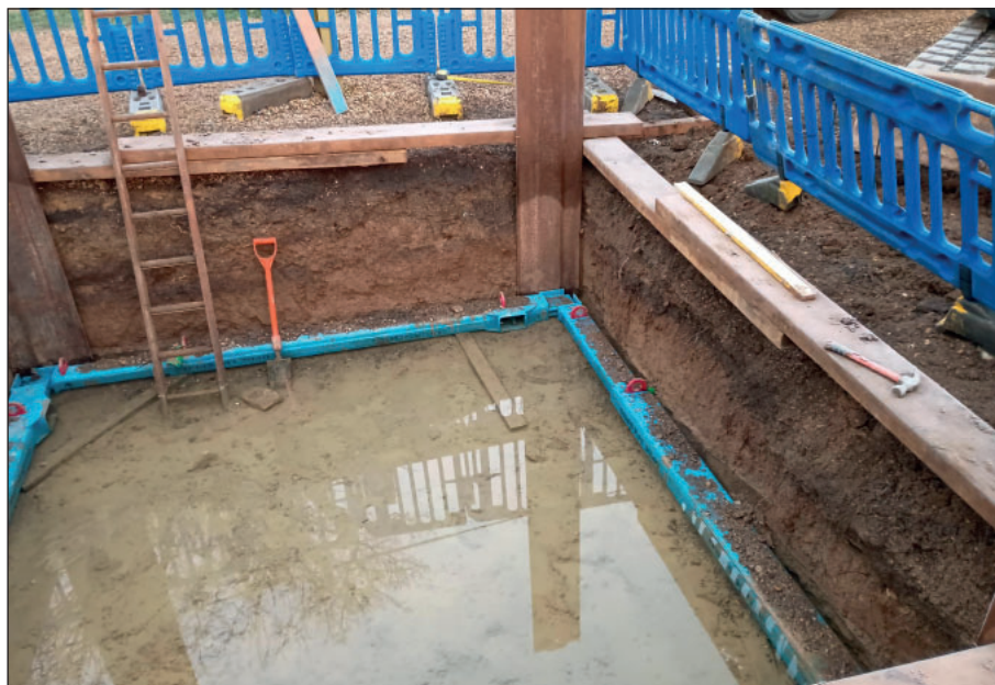
Figure 8. Trench 4 showing high level of groundwater
