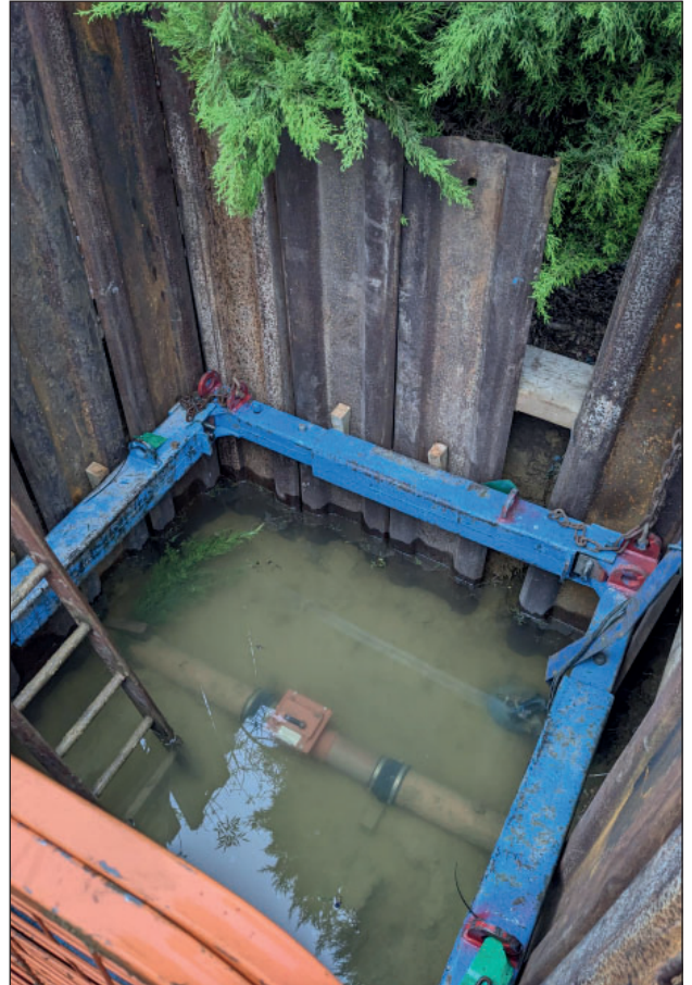
Figure 6. Trench 2 showing high level of groundwater
