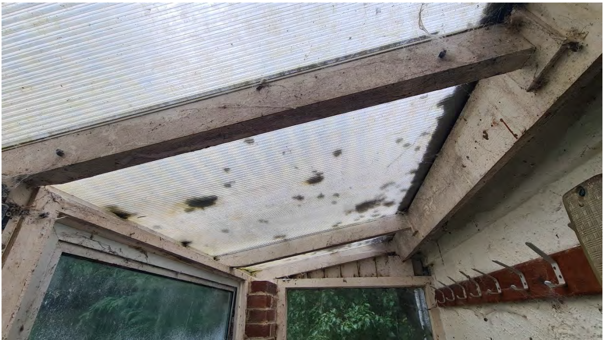
Plate 28 - Plastic corrugated roof of porch Room G1
