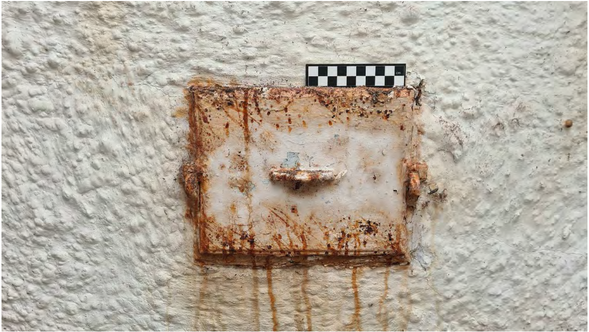
Plate 31 - Cast Iron soot door
