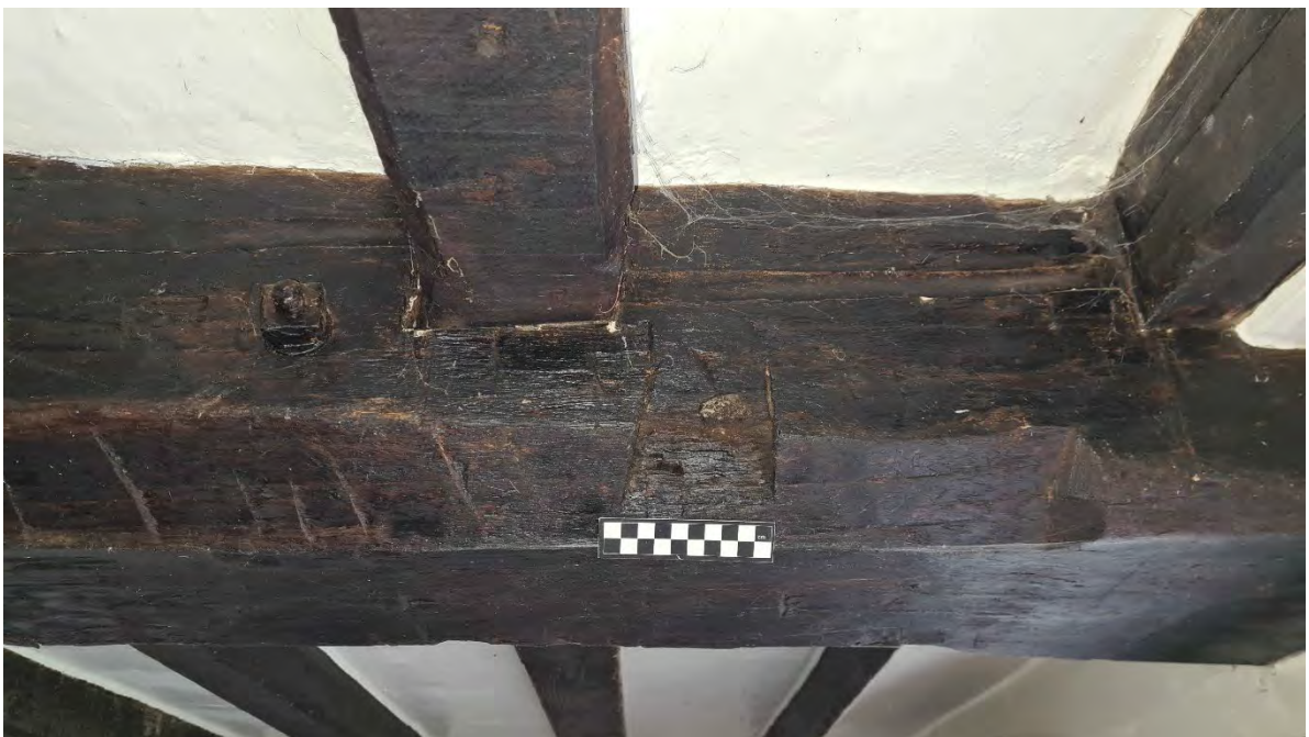
Plate 72 - South facing photo of timber and timber peg fitting beam in Room G7
