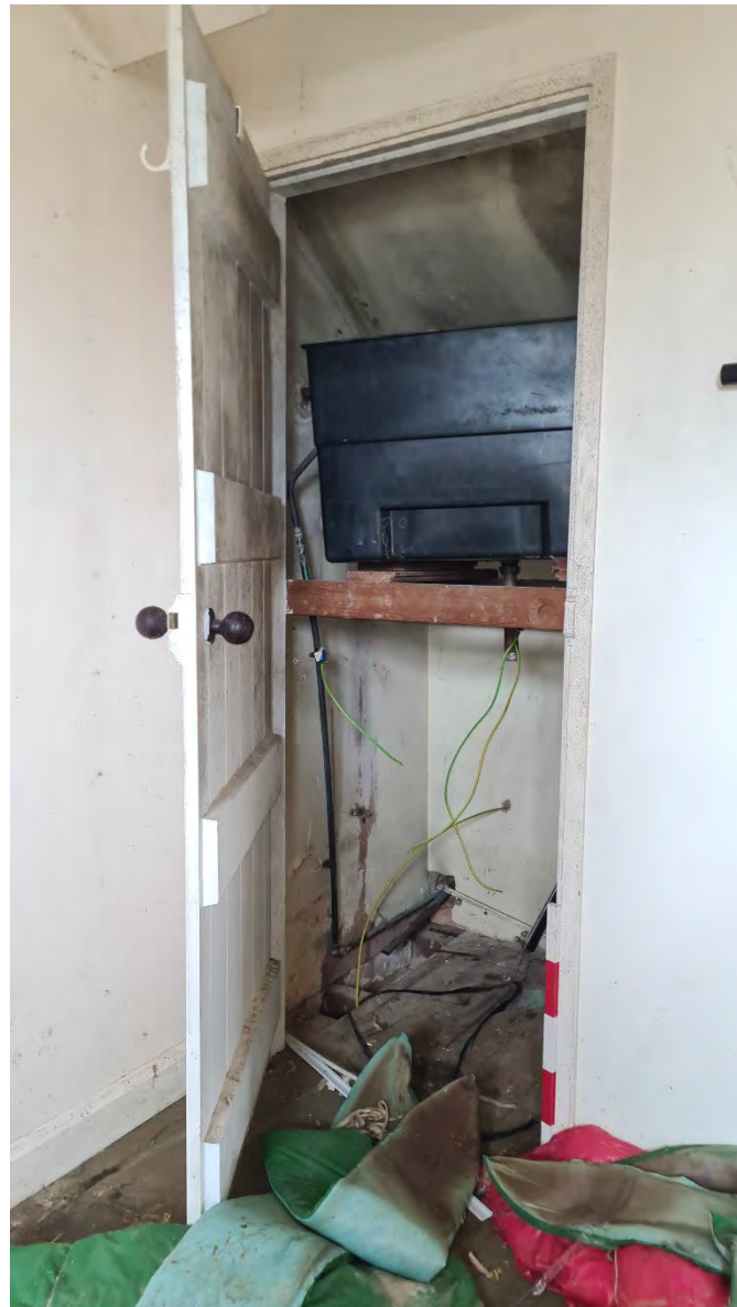
Plate 84 - Northwest facing photo of boiler Room G8
