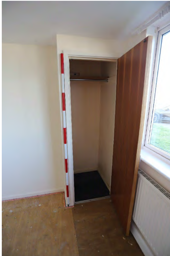
Plate 36 - North facing photo of modern storage cupboard in the south-east bedroom in bungalow 28
