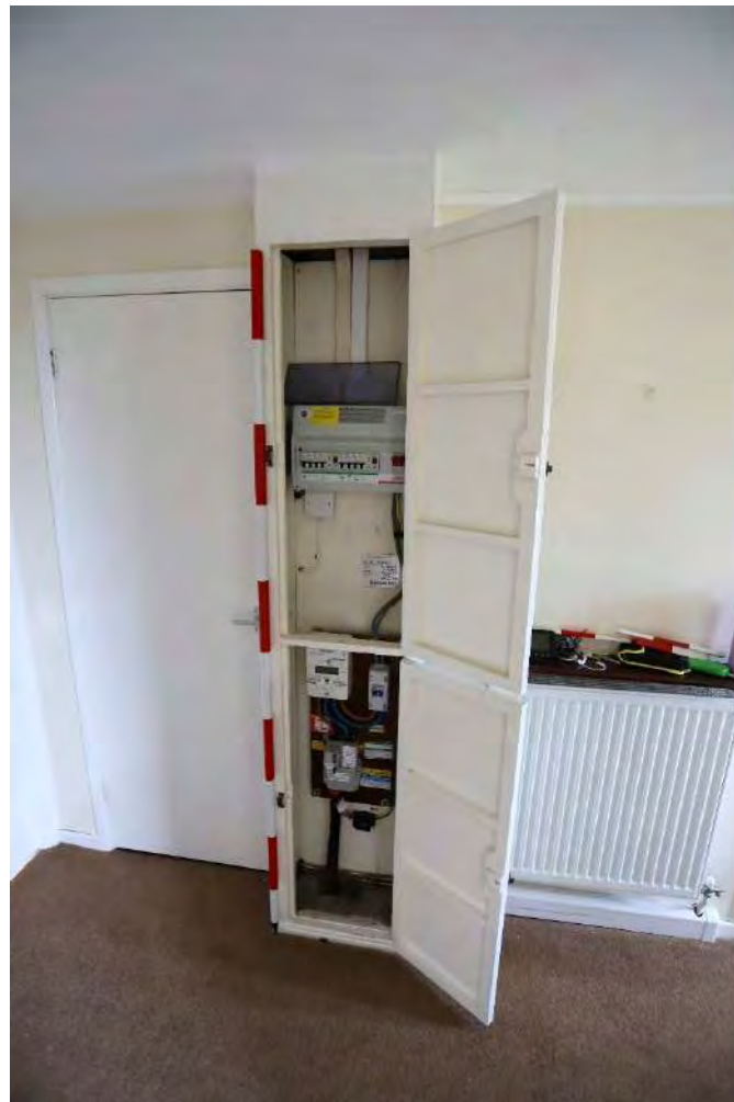
Plate 32 - North facing photo of utility cupboard in hallway of bungalow 43
