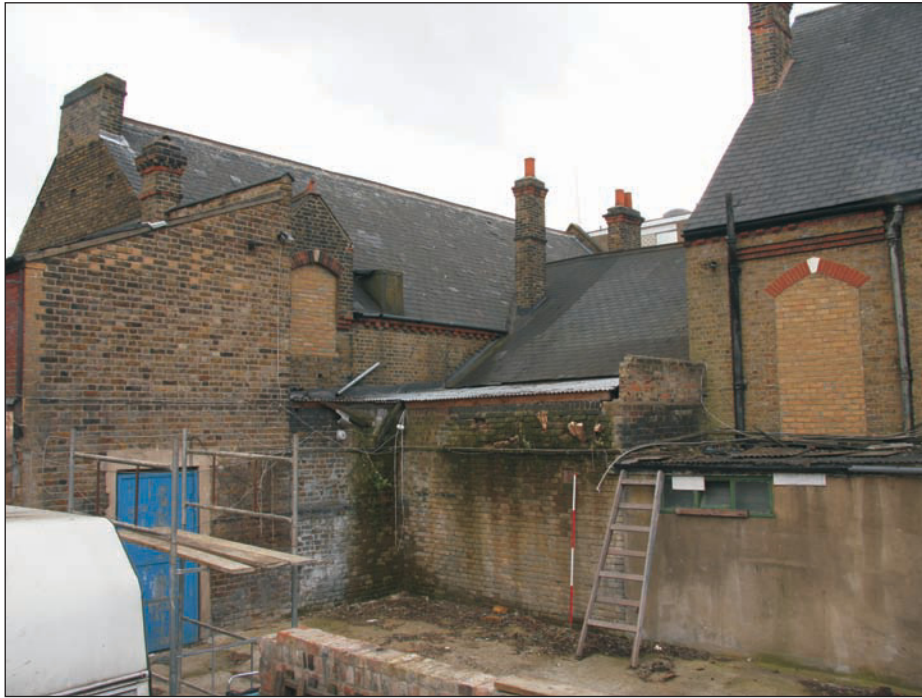
Plate 3: Partial view of northern elevation showing rear of link building and hall and corner of the main chapel. Looking south-east
