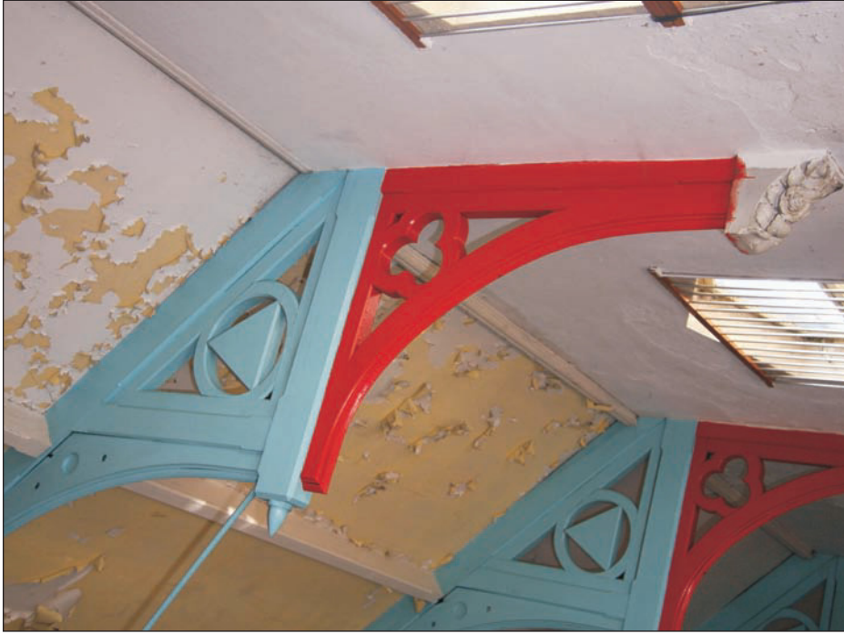
Plate 9: Detail of hammer beam and post supported by stone corbel, south interior wall of Main Worship Space. Looking south-east
