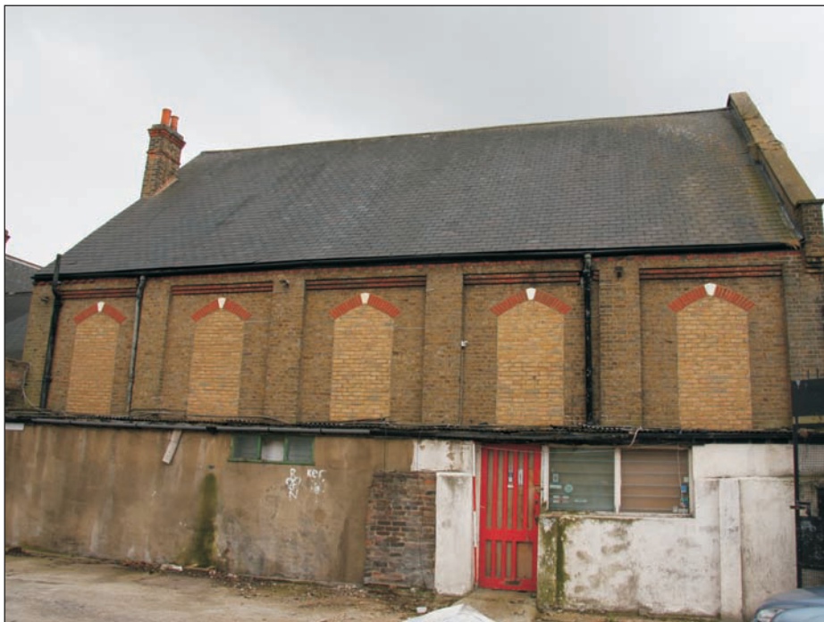
Plate 4: Northern elevation of Main Worship Space showing single storey lean-to. Looking south
