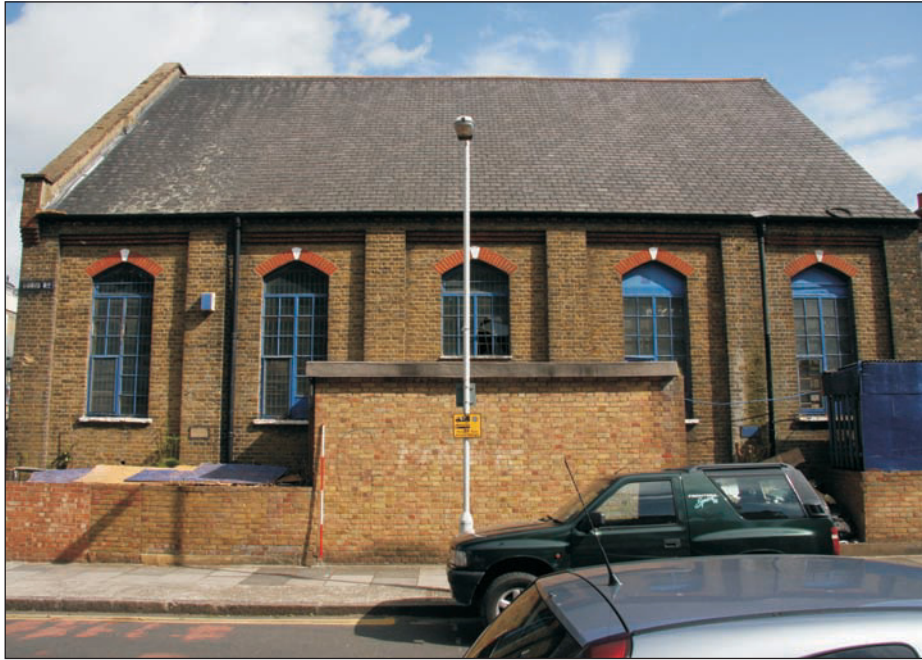
Plate 5: Southern elevation of Main Worship Space showing single storey lean-to. Looking north
