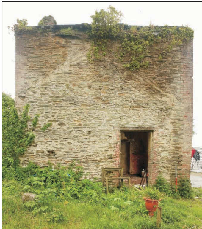
Plate 2: Two storey element A north elevation showing evidence of demolished north range
