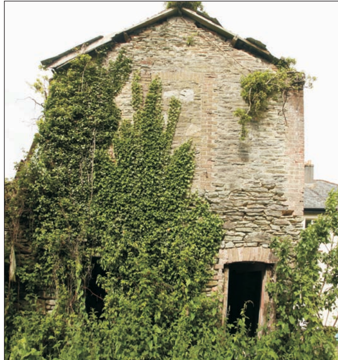
Plate 4: Two storey element A east facing elevation showing windows and blocked first floor door opening
