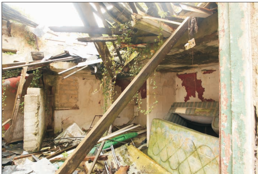
Plate 12: Series of low bays with concrete roof at south end of element B
