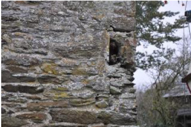
012: NORTHEAST ELEVATION, BUILDING 1: PATCHED 'HOLE'. SW FACING.
