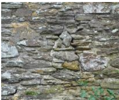
027: NORTHWEST ELEVATION, BUILDING 1: CRACKS AND PATCHING ABOVE WINDOW 6
