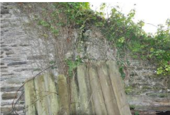
032: NORTHWEST ELEVATION, BUILDING 1 AND EXTENSION 1 SHOWING CRACKING BETWEEN THEM. SE FACING SHOT.
