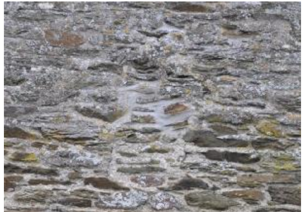
013: NORTHEAST ELEVATION: DETAIL OF PATCHING
