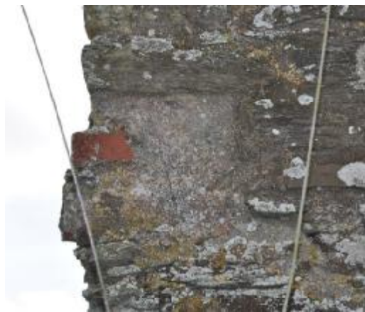
028: NORTHWEST ELEVATION, BUILDING 1: 'HOLE' ON SOUTHWEST CORNER
