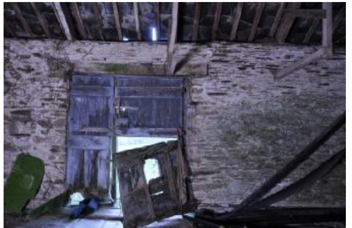
095: BUILDING 1, FIRST FLOOR INTERNAL: SW WALL, NW HALF AND DOOR 4, SW FACING.
