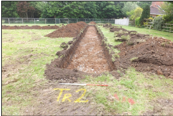
PHOTOGRAPH 1: TRENCH 2A LOOKING SOUTHWEST - TYPICAL SHALLOW TRENCH IN THE NORTHERN HALF OF THE SITE
