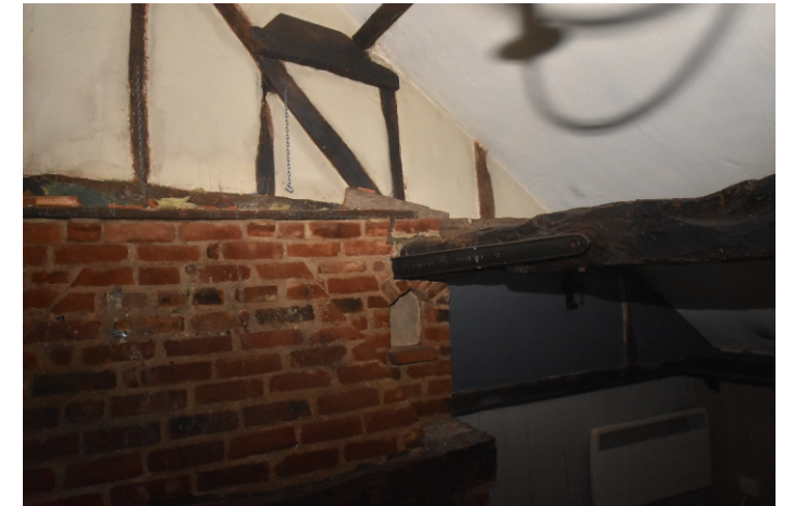
Plate 37: Room I, beam intruding into the fireplace
