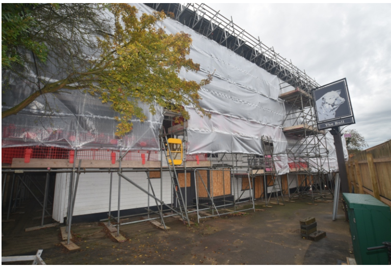
Plate 1: The front elevation of the Bull Hotel with scaffolding and sheeting cover
