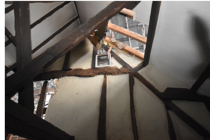
Plate 36: Room I rear wall, purlin with a 'V-shaped' cut-out showing the position of the original purlin
