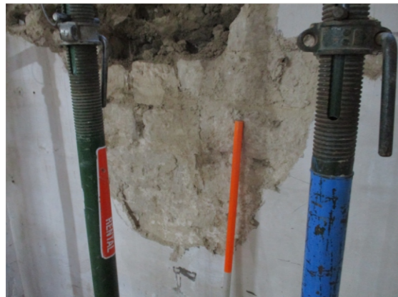
PHOTOGRAPH 9: INTERIOR WALL STONES, EXPOSED AFTER REMOVAL OF WALL RENDER
