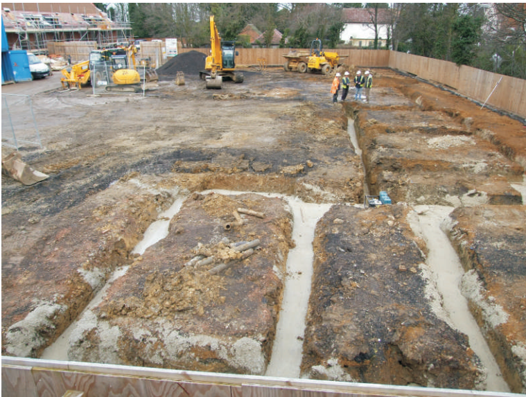
NORTH FACING SHOT OF PLOTS 55 AND 54, 55 EXCAVATED AND CONCRETED AND 54 PREDOMINANTLY EXCAVATED.
