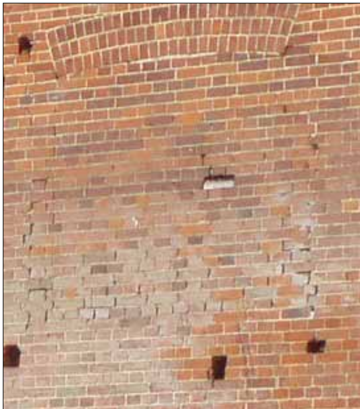
Plate 4: Blocked up window
