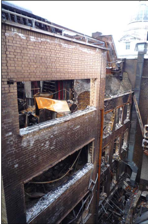
Plate 11 Fire-damage rear elevation viewed to south-west
