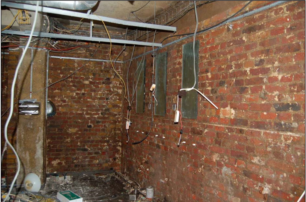
Plate 19 Historic east wall of nos. 5-7 and rear (north) wall of nos. 9-11 viewed in basement
