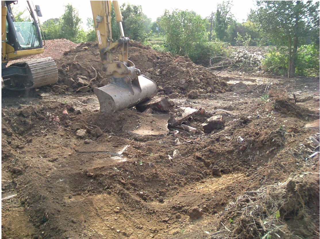
Plate 1 Removal of floor slabs, yard area and drains to former Porters Hall Cottage
