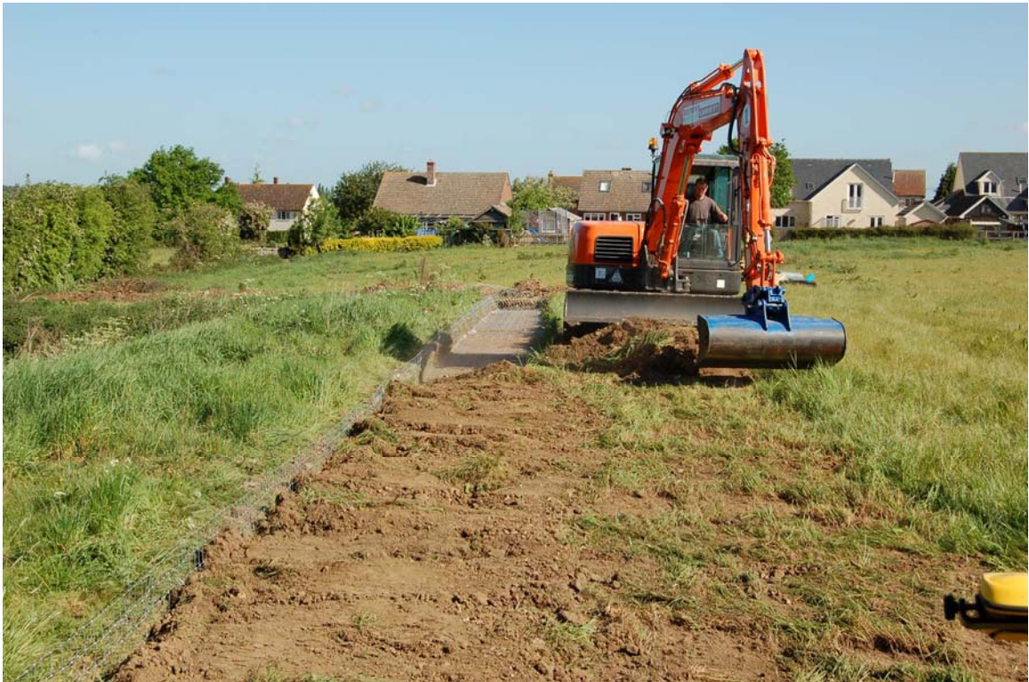
Plate 4 Trench (as above) being backfilled after the fencing has been laid in it. The upstanding wire on the right will link to the vertical section of the fence
