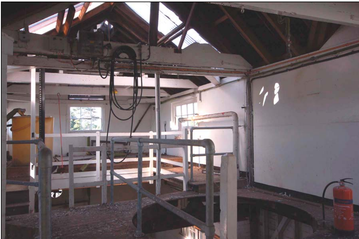
Plate 59 Second floor viewed towards former hop back and south-east gable of tower block
