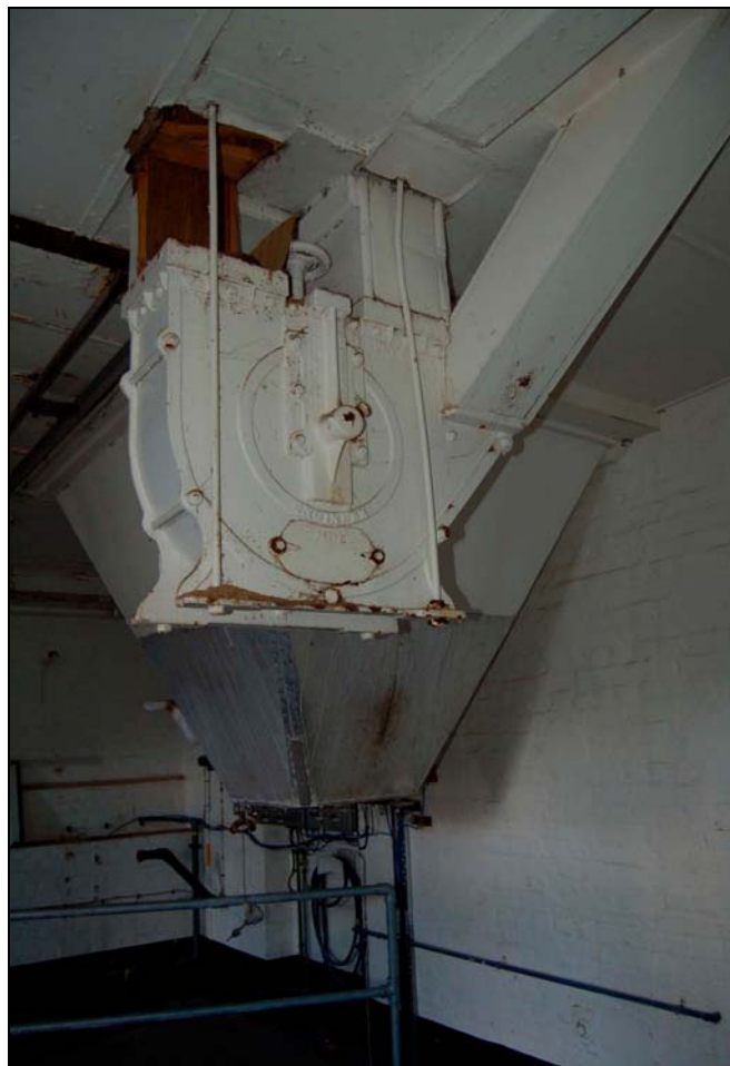
Plate 49 Base of Bobby elevator in mashing room
