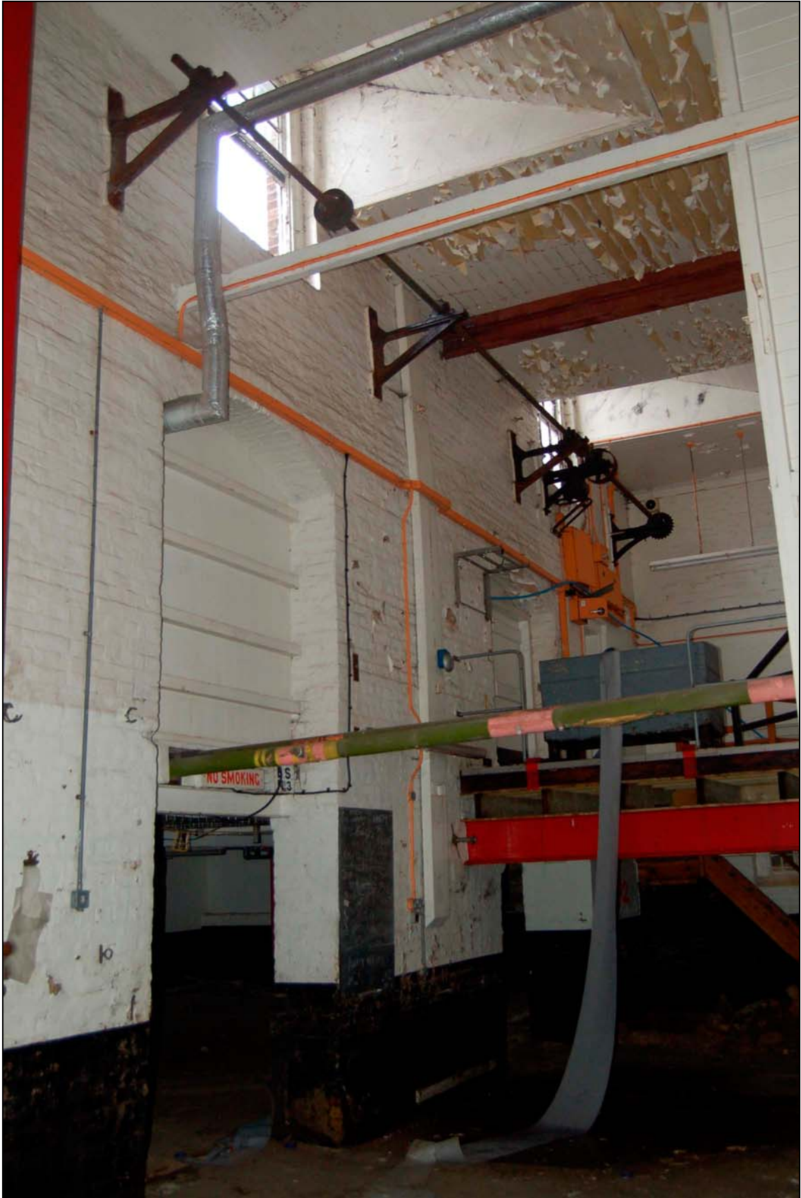
Plate 37 Line-shafting for cask hoists viewed to north
