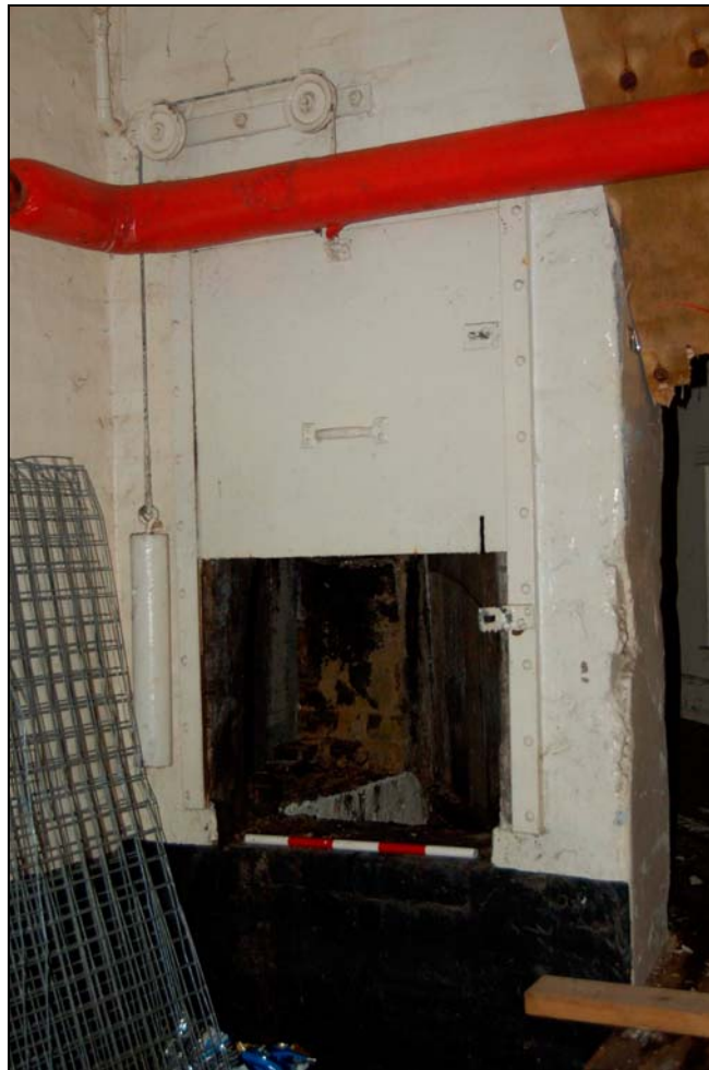
Plate 34 Maintenance door for vertical line-shaft in loading area
