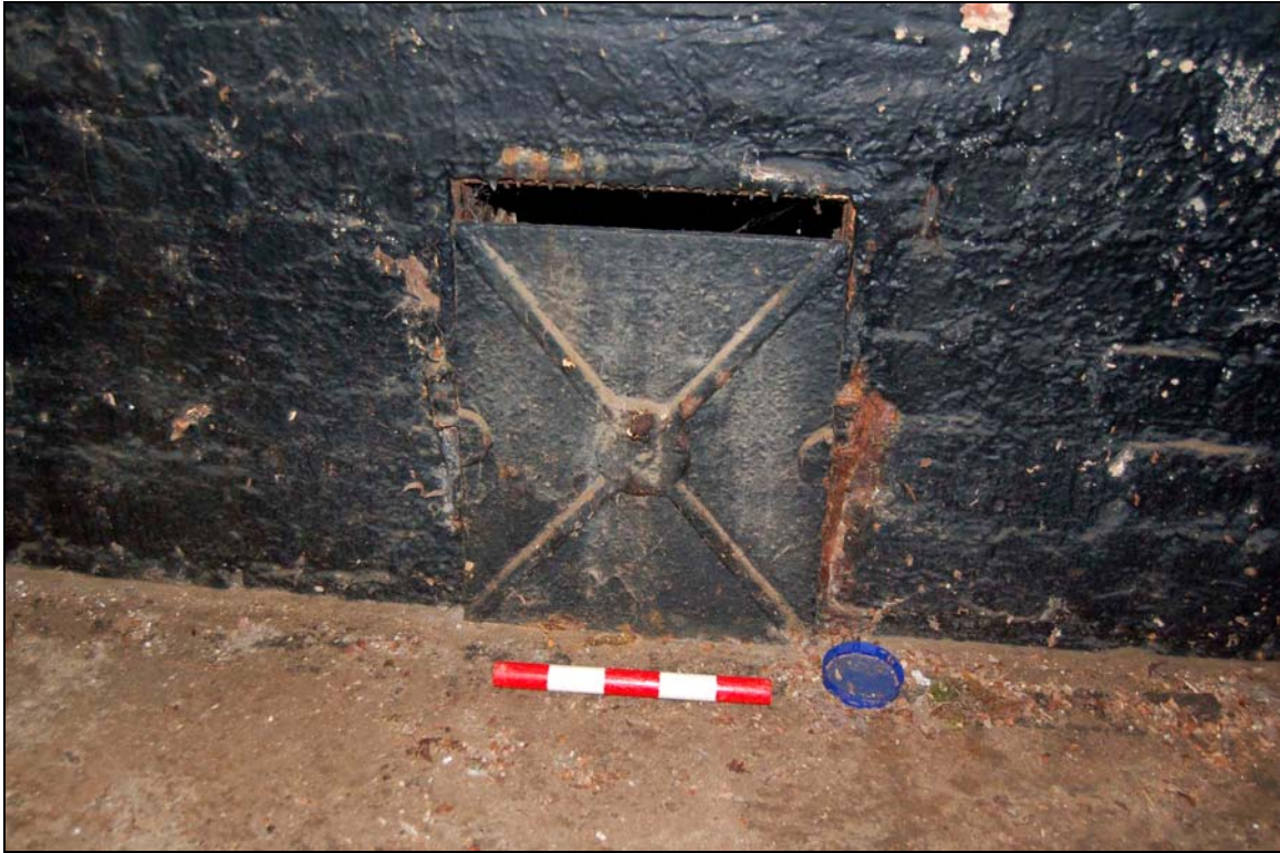
Plate 29 Metal plate in engine room (25cm scale)
