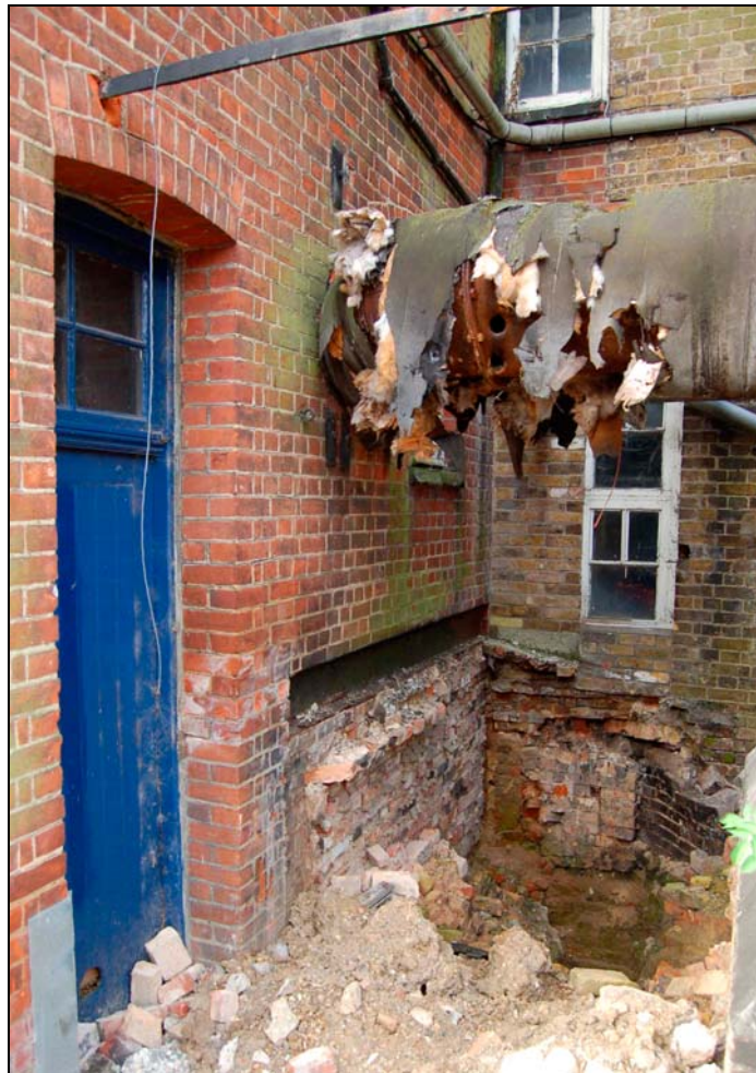
Plate 8 Blocked chimney flues from boiler house and engine house
