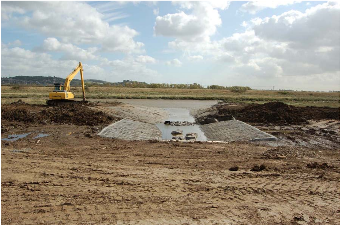
Plate 6 Completed structure. Looking from the saline lagoon embankment to Easthaven Creek at low tide.
