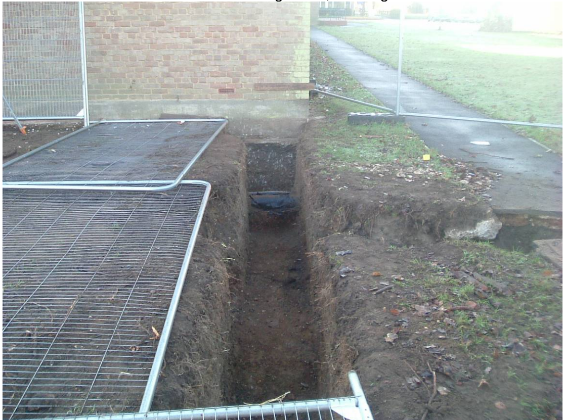
Plate 2: View of extension end wall looking WNW, showing service runs and drains
