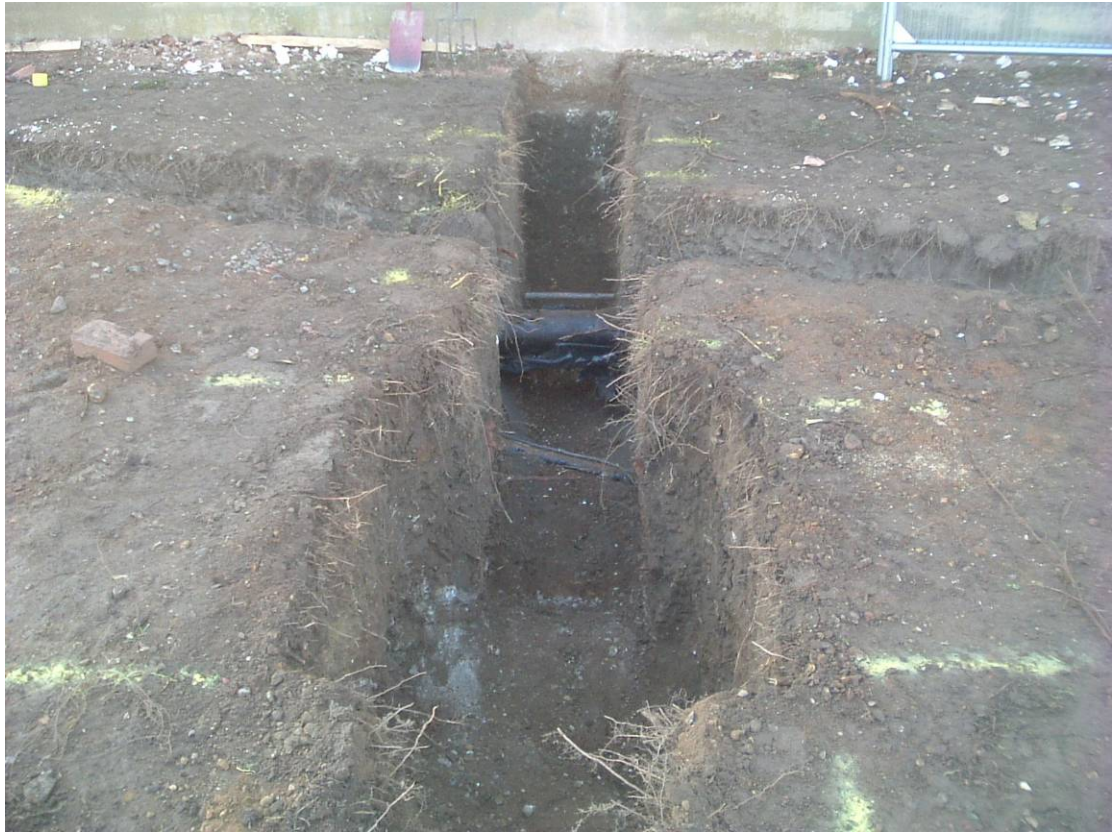
Plate 3: Foundation trench for dividing wall between Changing Rooms and Dance Studio showing service and former drain runs
