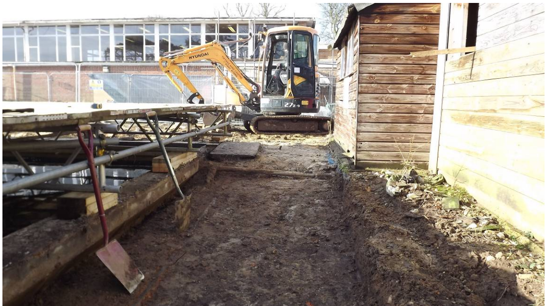
Plate 4: Pool works in progress – stripping of shallow trench for new concrete slab to support canopy
