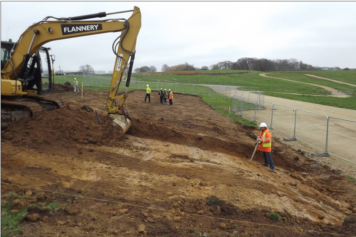
Plate 2. Re-profiling the existing ground level in the Accredited Stand area, looking northeast
