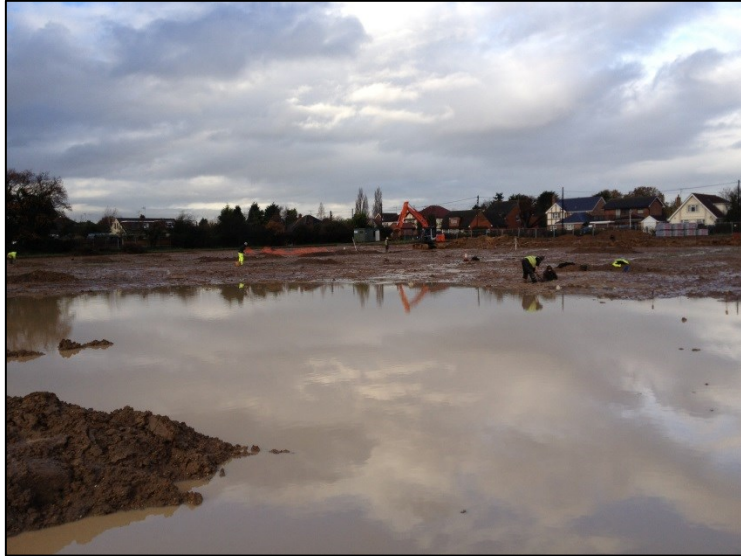
Figure 9. Excavation area flood conditions
