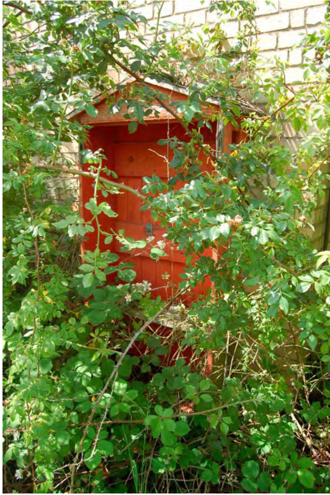
Plate 165 Fire point on east wall of garage
