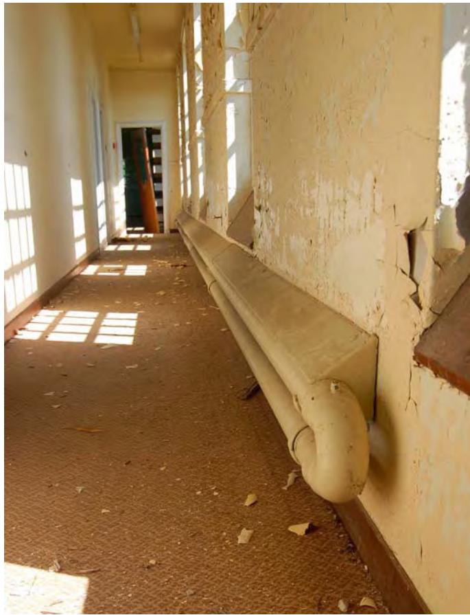
Plate 71 Shrouded heating pipes
