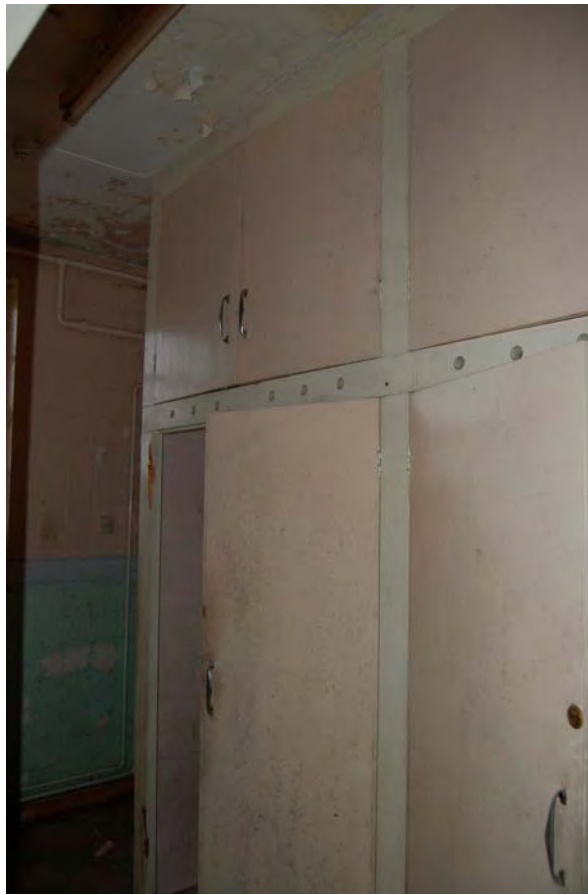
Plate 69 Cupboards in ablution block
