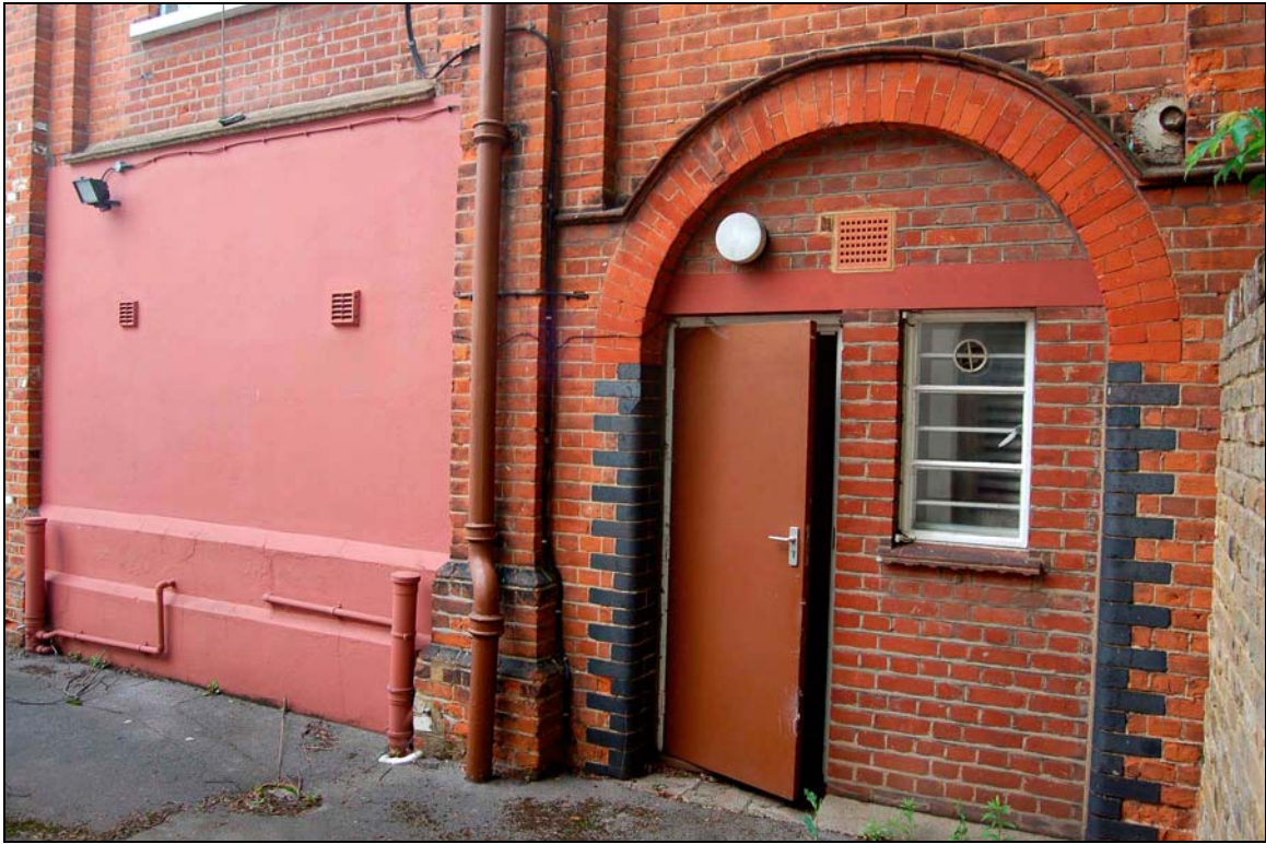
Plate 21. Blocked entrance on east side of pump house
