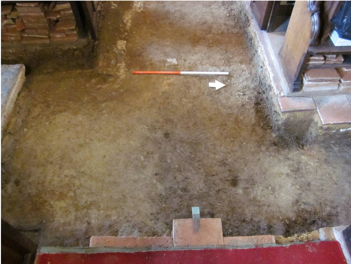
Plate 7. Mortar bedding for earlier floor in Nave Aisle, looking west (1m scale)
