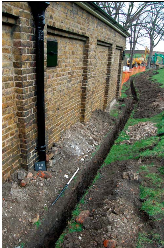
Plate 4 Brick pier 8 and rear wall of Artillery Store viewed to north-east (1m scale)
