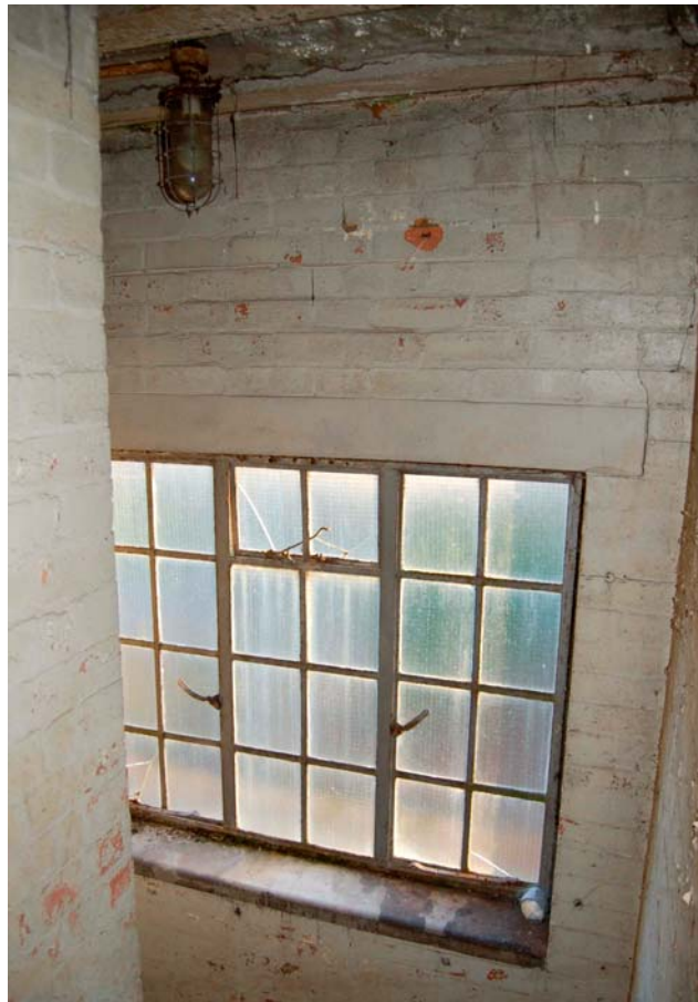
Plate 12 WW2 light fitting and Crittalls window
