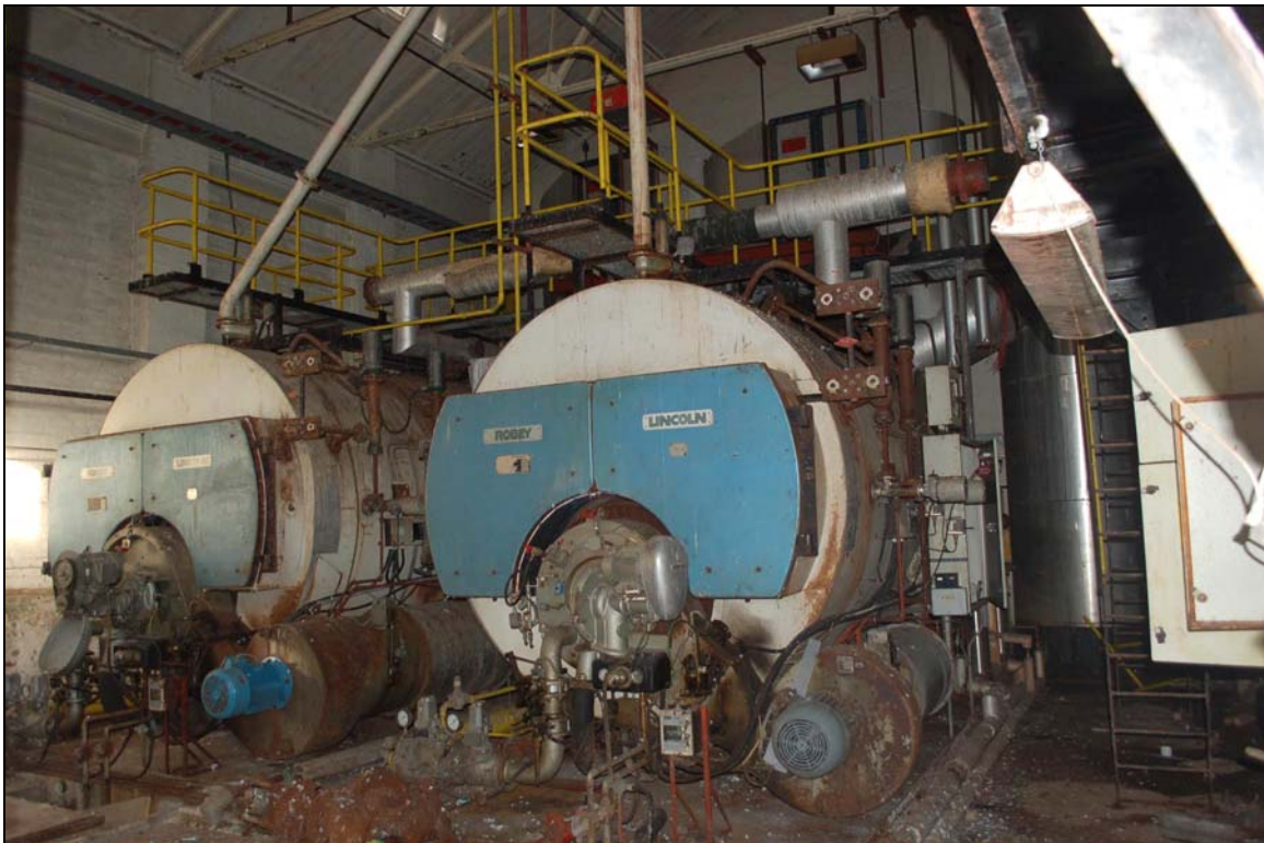
Plate 128 Robey boilers inside boiler room
