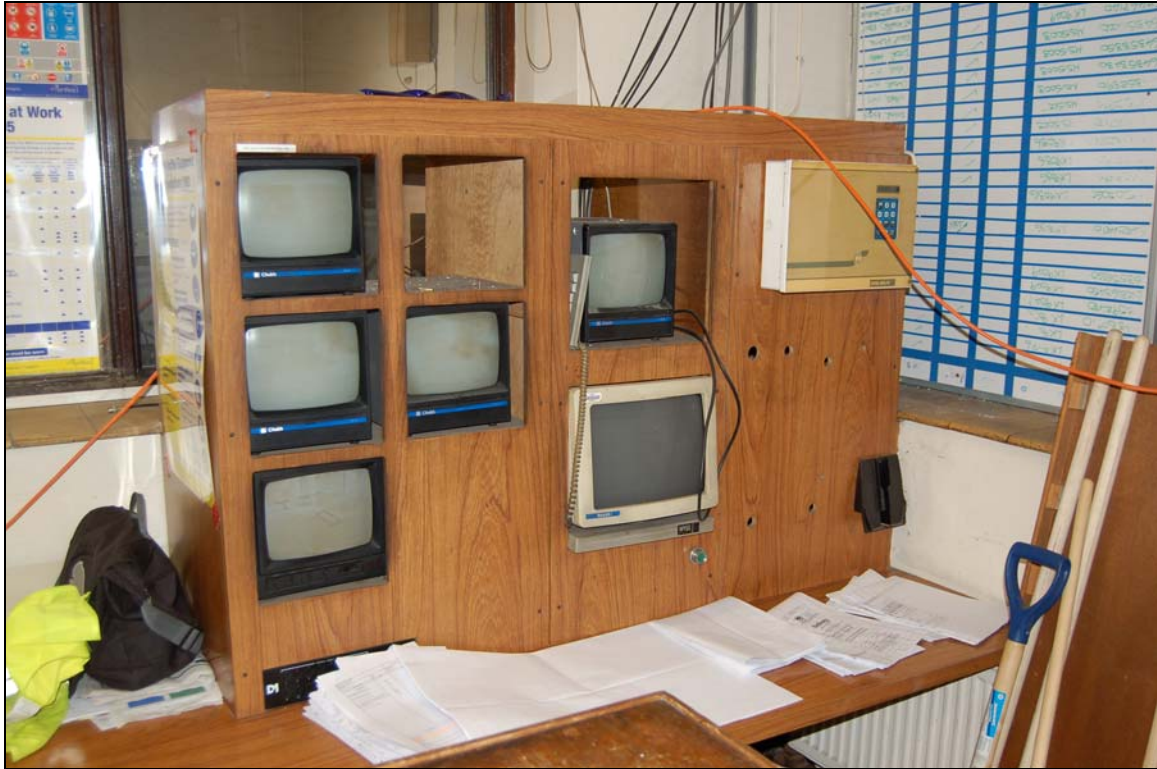
Plate 35 Monitors in control room 3
