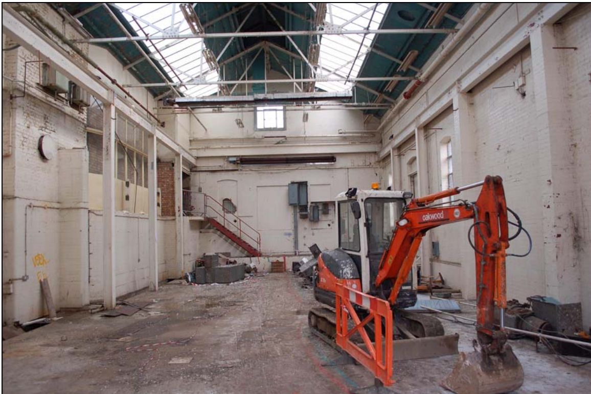
Plate 132 Generator room viewed to east
