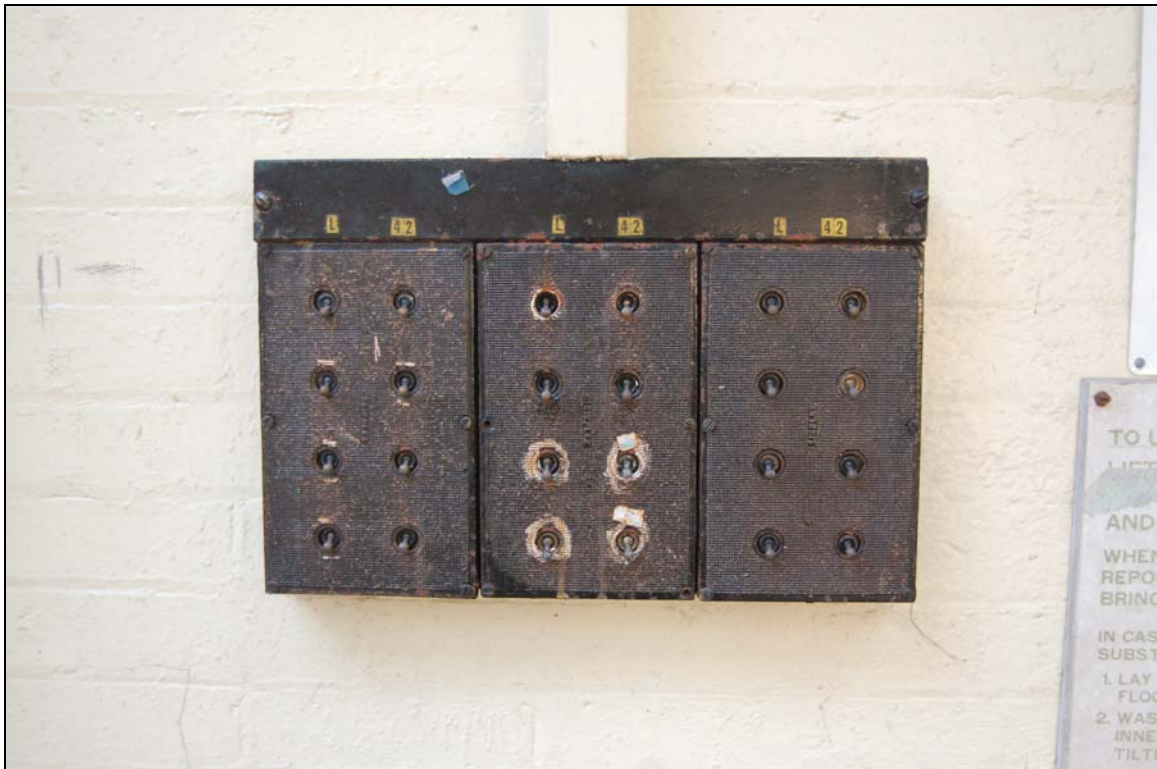
Plate 48 Electric light switch board
