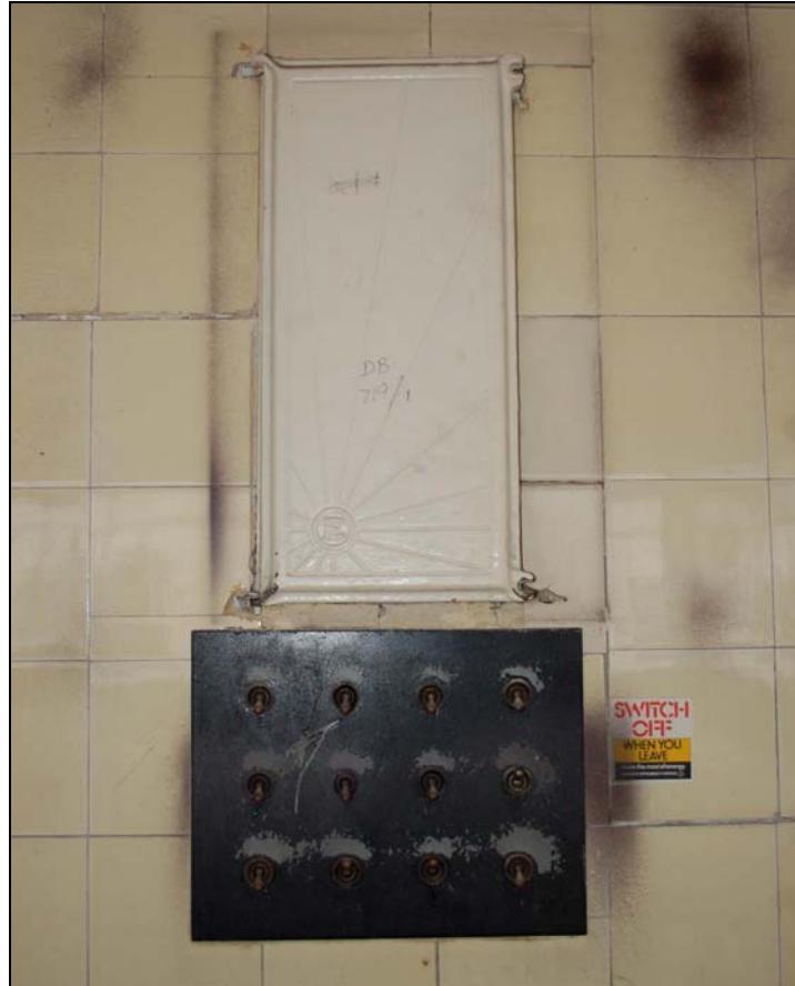
Plate 123 Switch board on south wall of canteen 1
