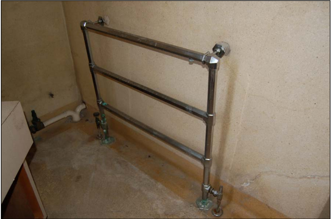
Plate 101 Art-Deco style radiator in washroom on fourth floor
