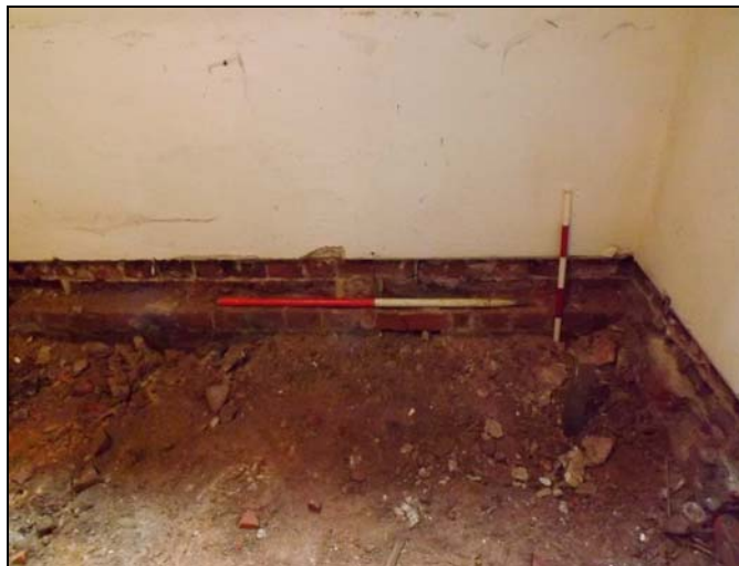
Plate 3: Detail showing depth of cavity beneath timber flooring, looking south. (1 and 0.5m scale).
