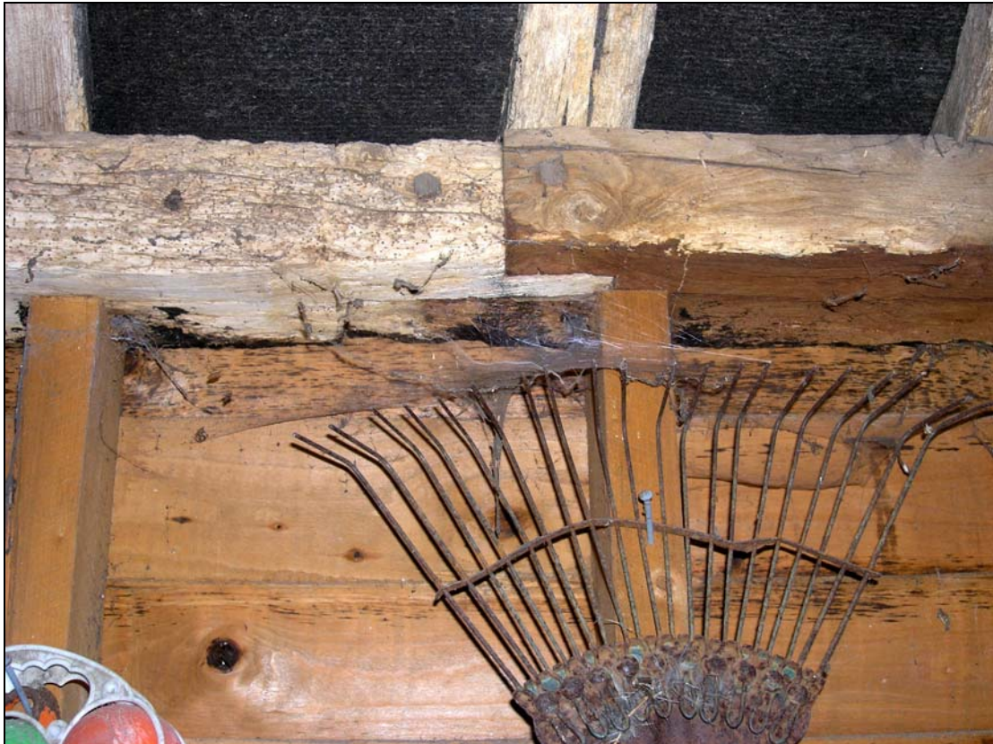
Plate 8 Edge-halved and bladed scarf jointed wall plate above in-filled wall framing in Shed 1
