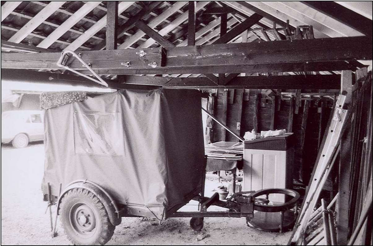
Plate 19 King post trusses and internal north-west side of timber partition to Shelter Shed 4
