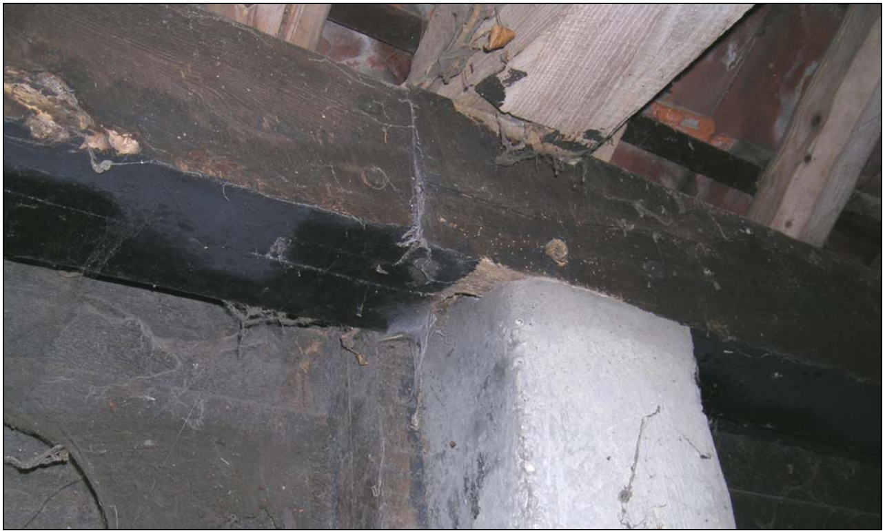
Plate 10 Concrete bay post partly obscuring empty mortise on wall plate soffit. Edge-halved and bladed scarf joint over
