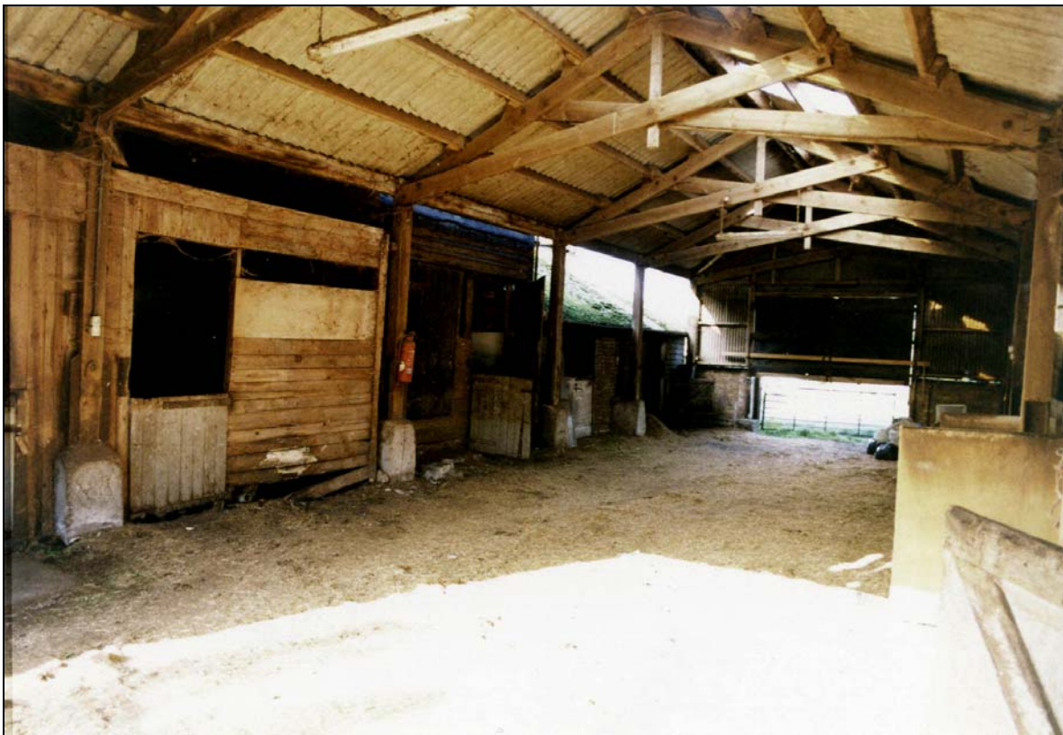
Plate 4 Interior of Covered Yard & stables either side of Barn porch, viewed from south-east
