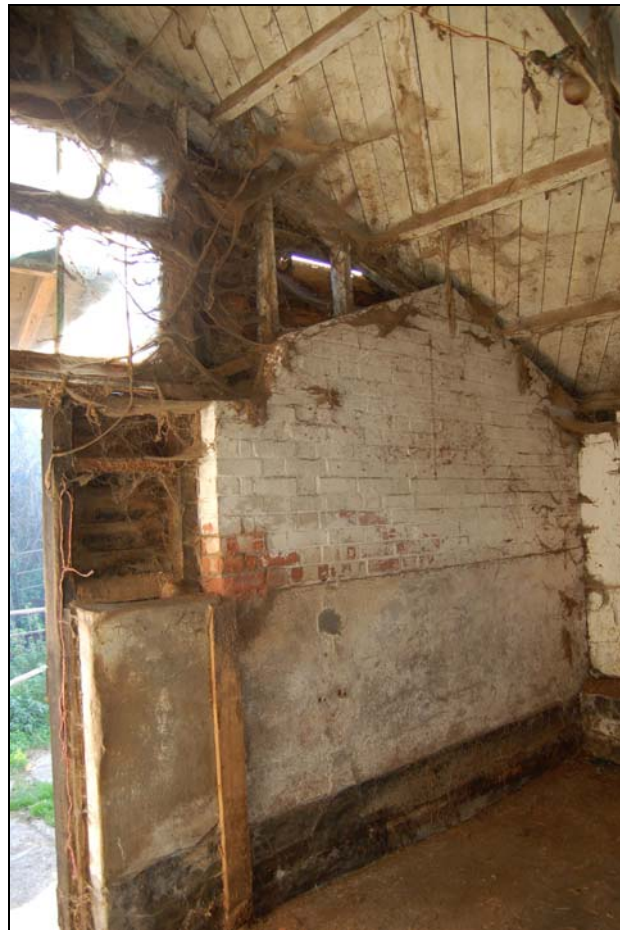
Plate 20 Gable to earlier brick structure preserved within south wall of Stable 2c
