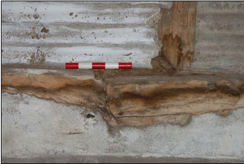
Plate 11 Bridle scarf joint with squinted abutments and over-lipped face in ground sill
