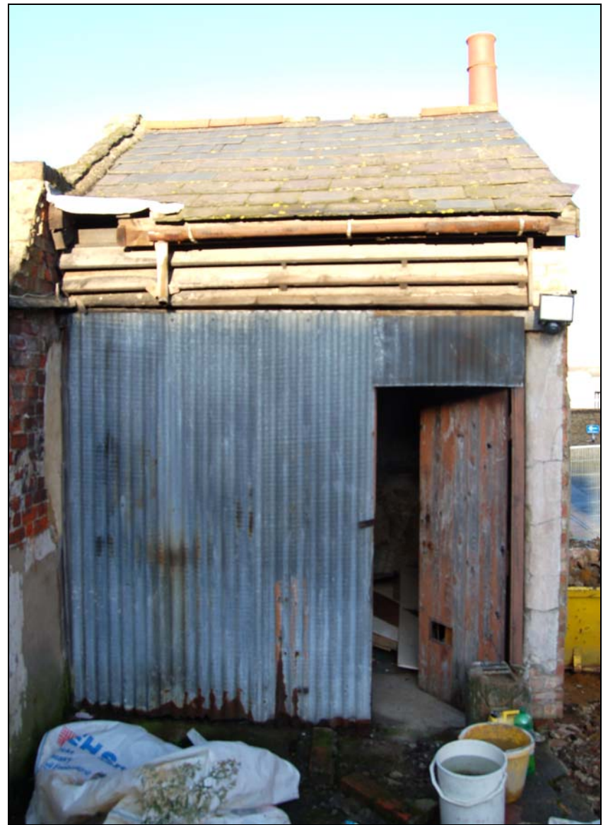
Plate 4 Inserted corrugated iron wall below main smoke vent
