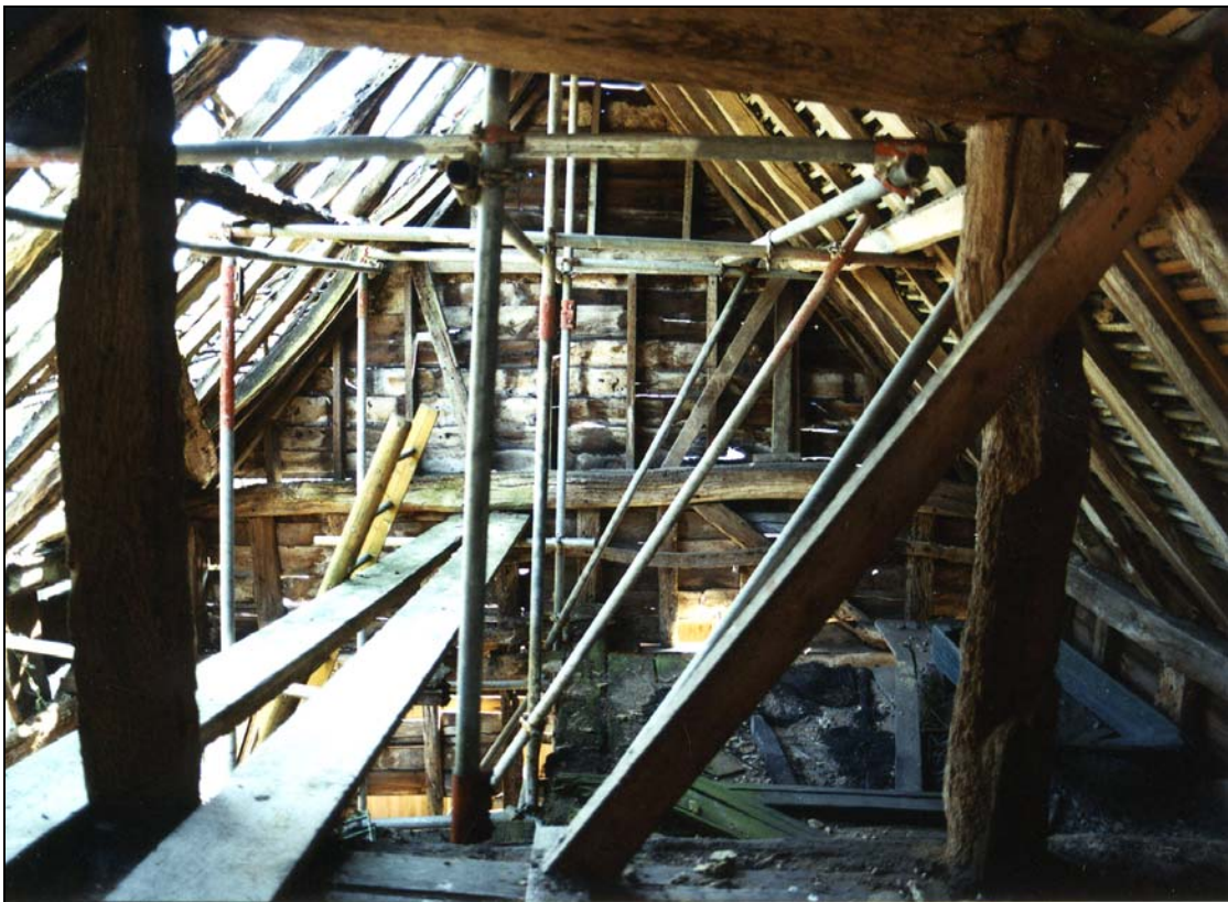
Plate 22 View through queen post truss across first floor of byre to rebuilt south gable
