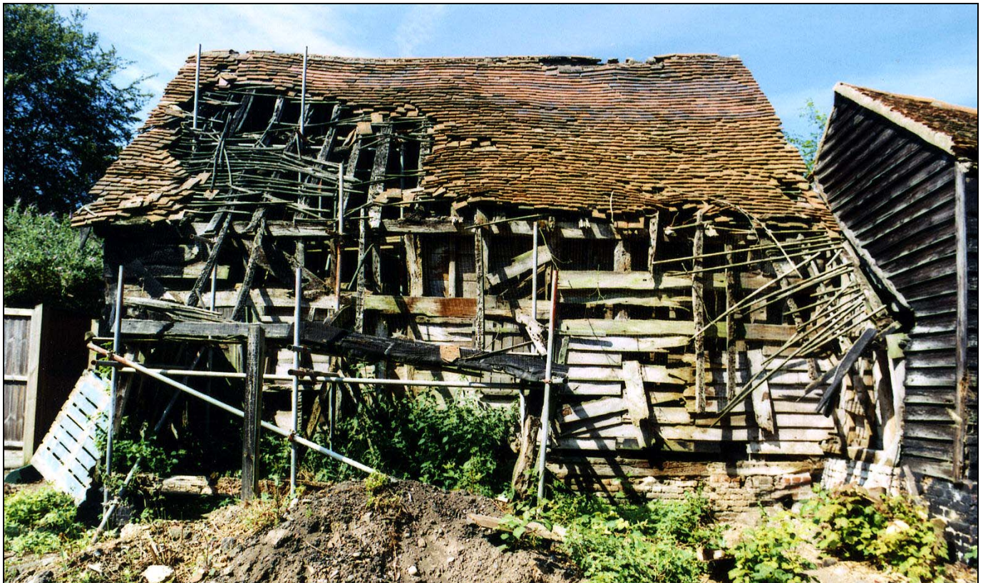
Plate 14 Dilapidated rear of byre viewed from east
