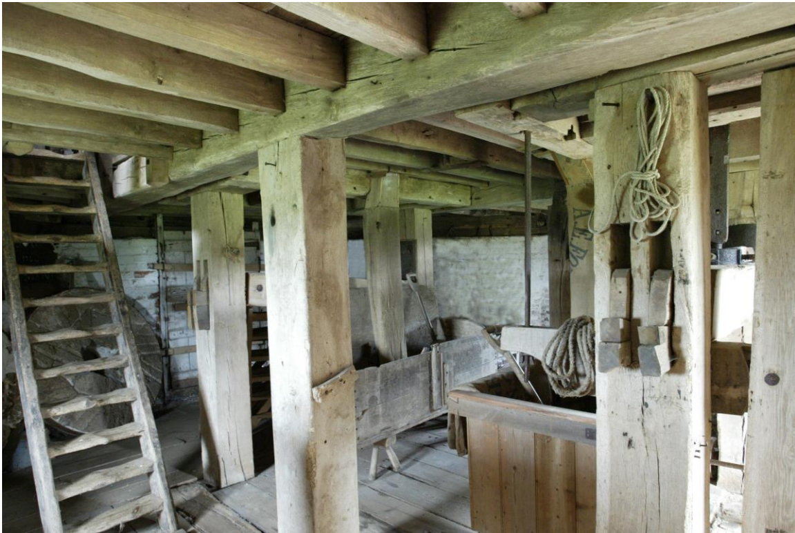
Plate 6. The substantial timber frame or 'hurst' supporting the millstones and machinery on the stone floor of the early 19th-century smock mill at Lacey Green, near Princes Risborough, Bucks. (Reproduced by permission of the Chiltern Society ©)
