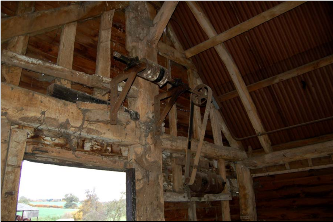
Plate 11 Former motor and drivebelts for grain processing in barn 1a
