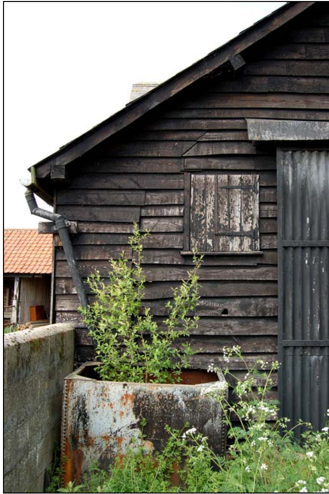
Plate 5 Scar to former roof line on east elevation
