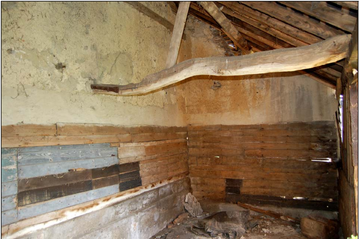
Plate 12 External walls of barn & porch viewed from interior of loose box 1a
