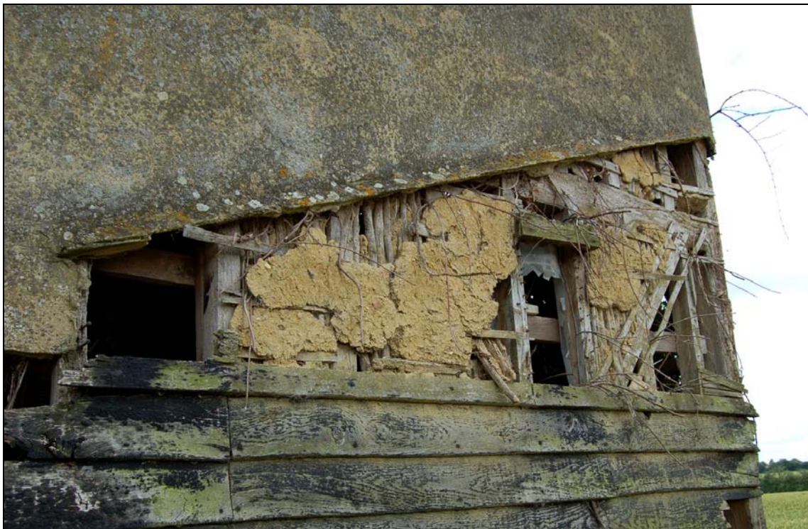
Plate 6 Exposed daub render to barn within wall scar to former north range
