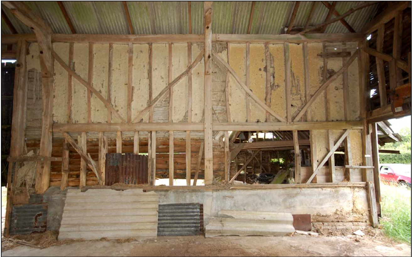
Plate 15 Detail of wall framing south of threshing floor, on east side against byre
