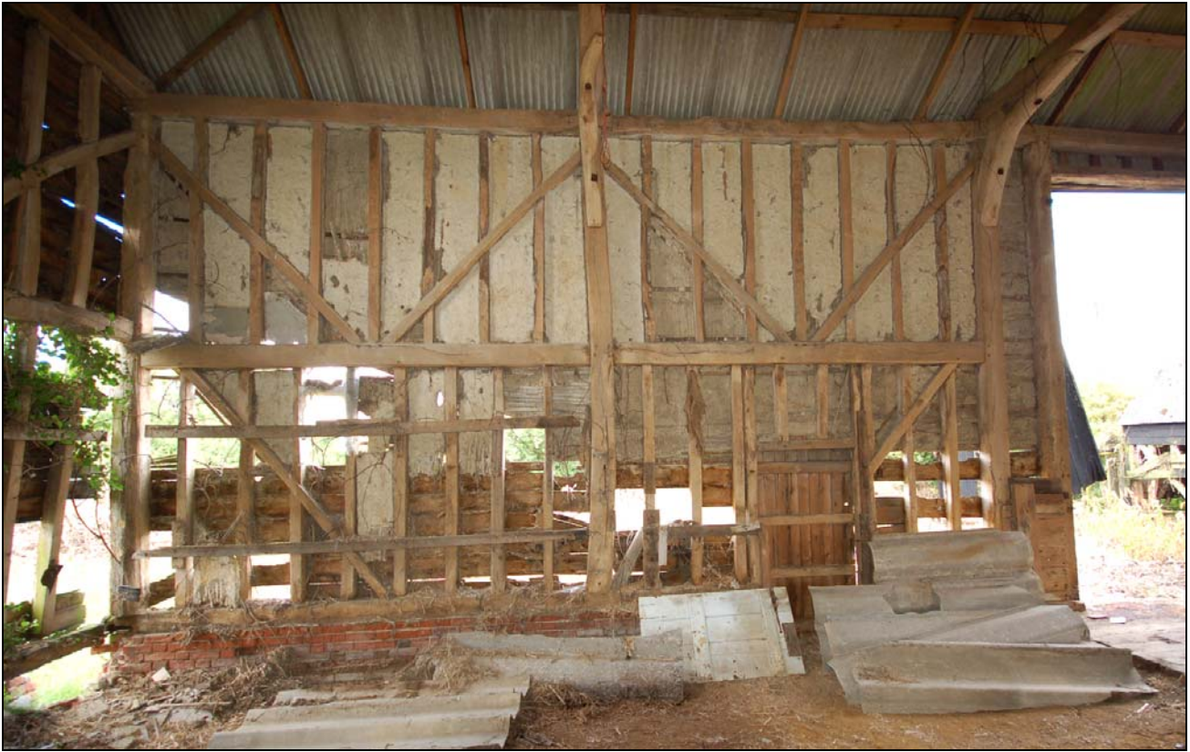
Plate 13 Wall framing and ground sill scarf joint on northern bays, east wall
