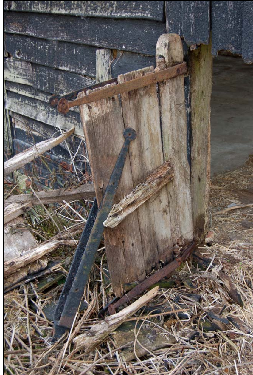
Plate 4 Detail of leap door on east side
