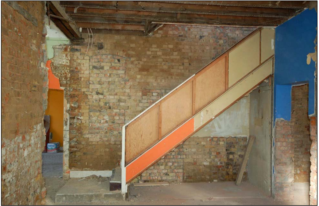
Plate 19 Blocked areas in partition wall between engine house and south part of office range
