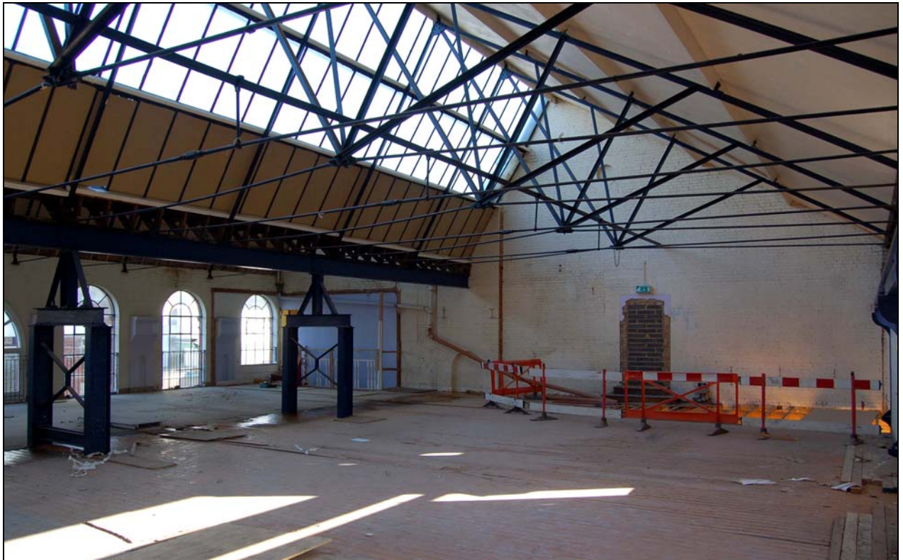
Plate 14 Blocked doorway cut through blocked window on east wall of engine house
