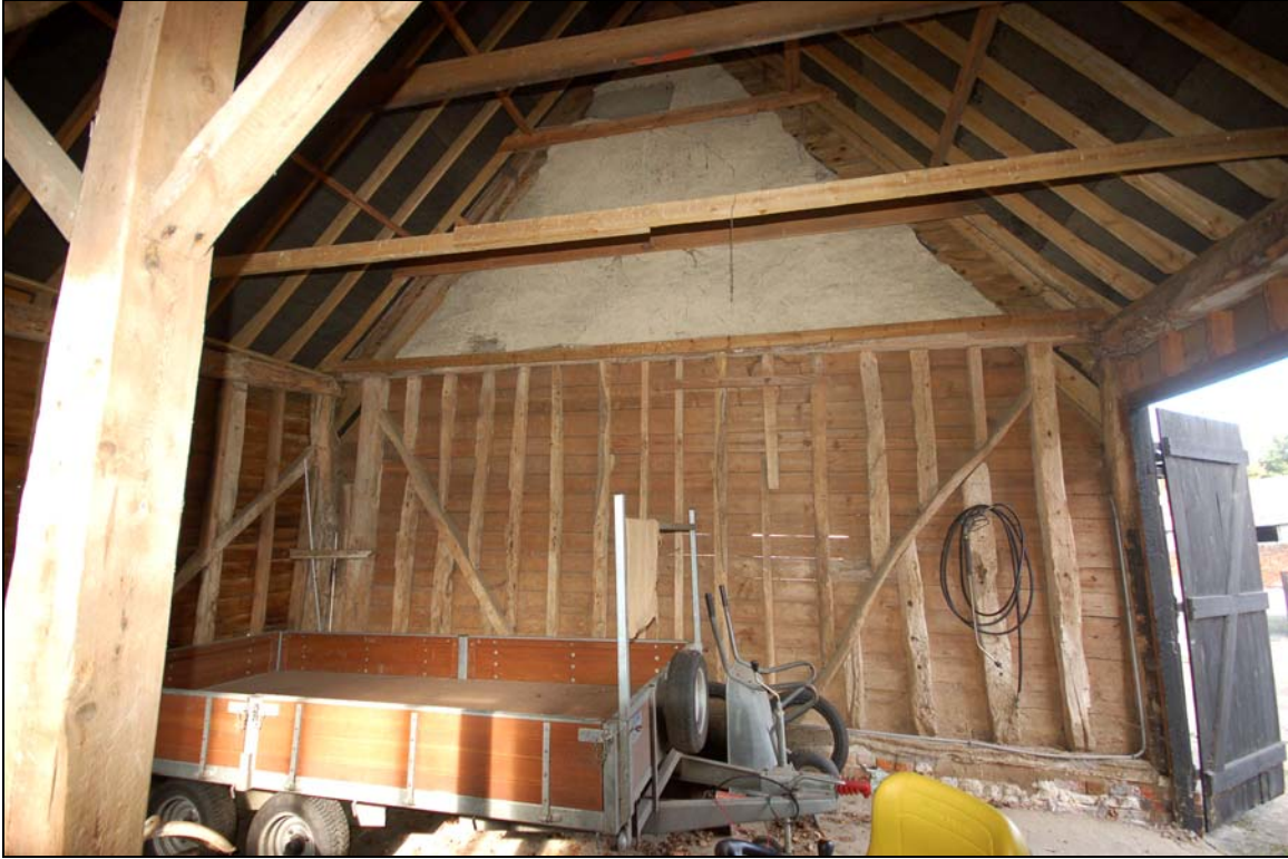
Plate 39 Extant lime plastered partition wall between machine store 9 & granary 10 & former roof line of missing end
