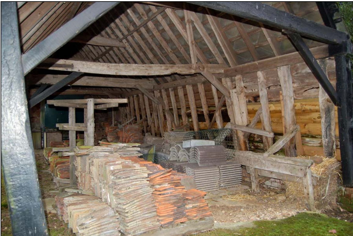
Plate 36 Interior of shelter shed 8 viewed to east from missing bay
