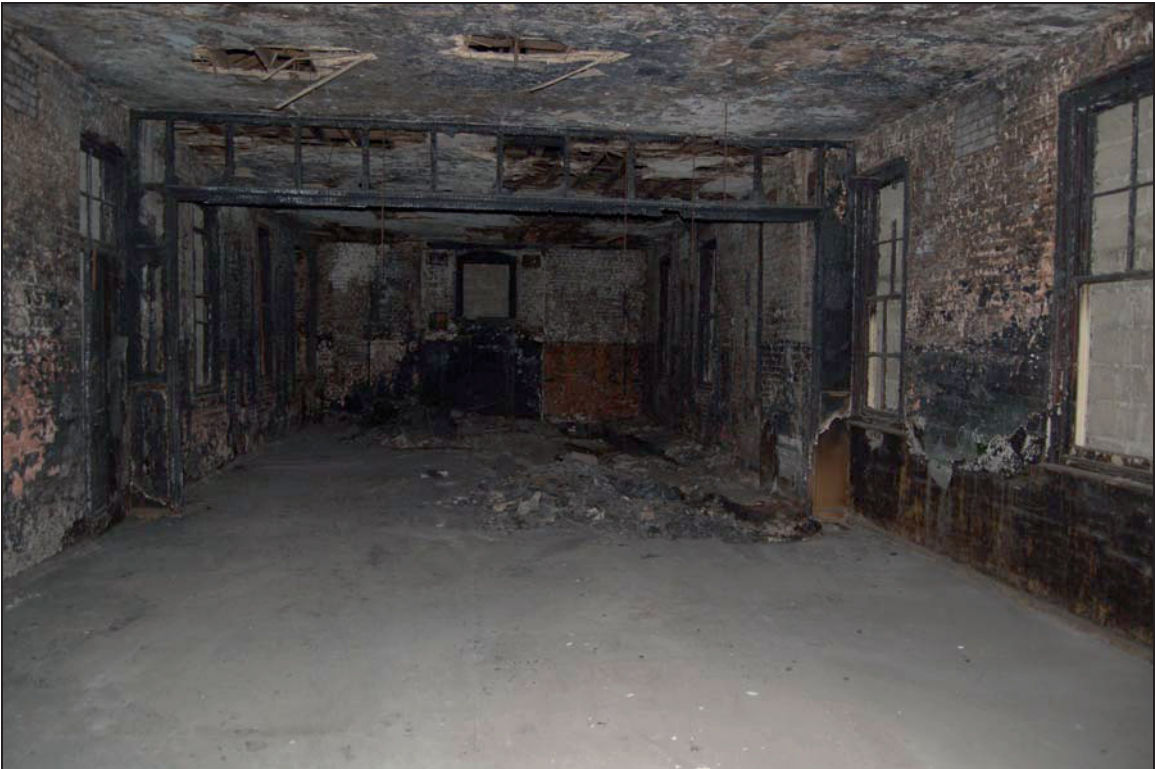
Plate 18 Interior of fire-damaged barrack room
