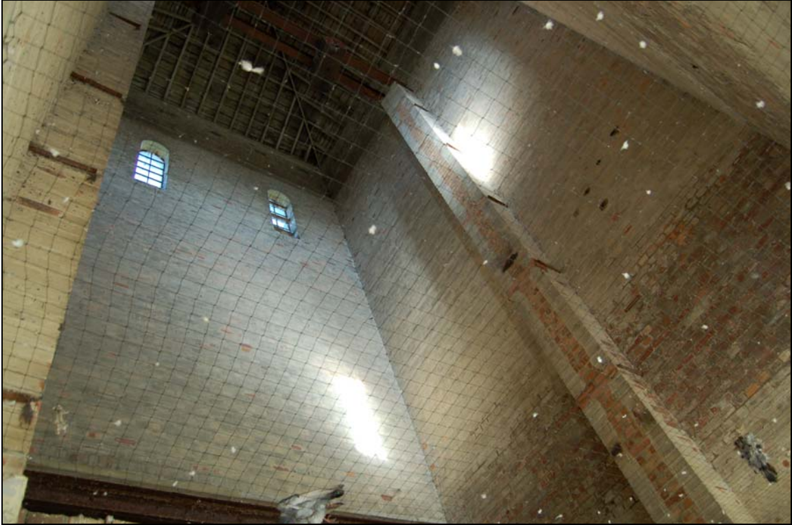
Plate 19 Inside the accumulator tower
